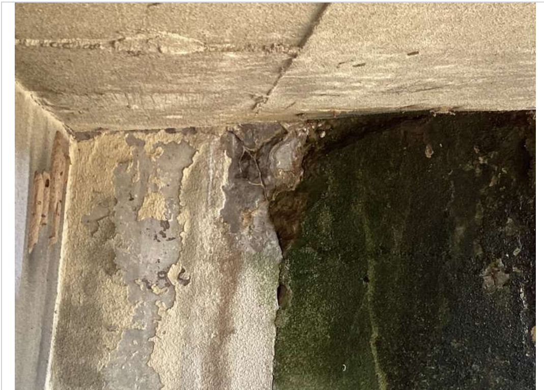
Abutment 2 spall on backwall under right overhang
