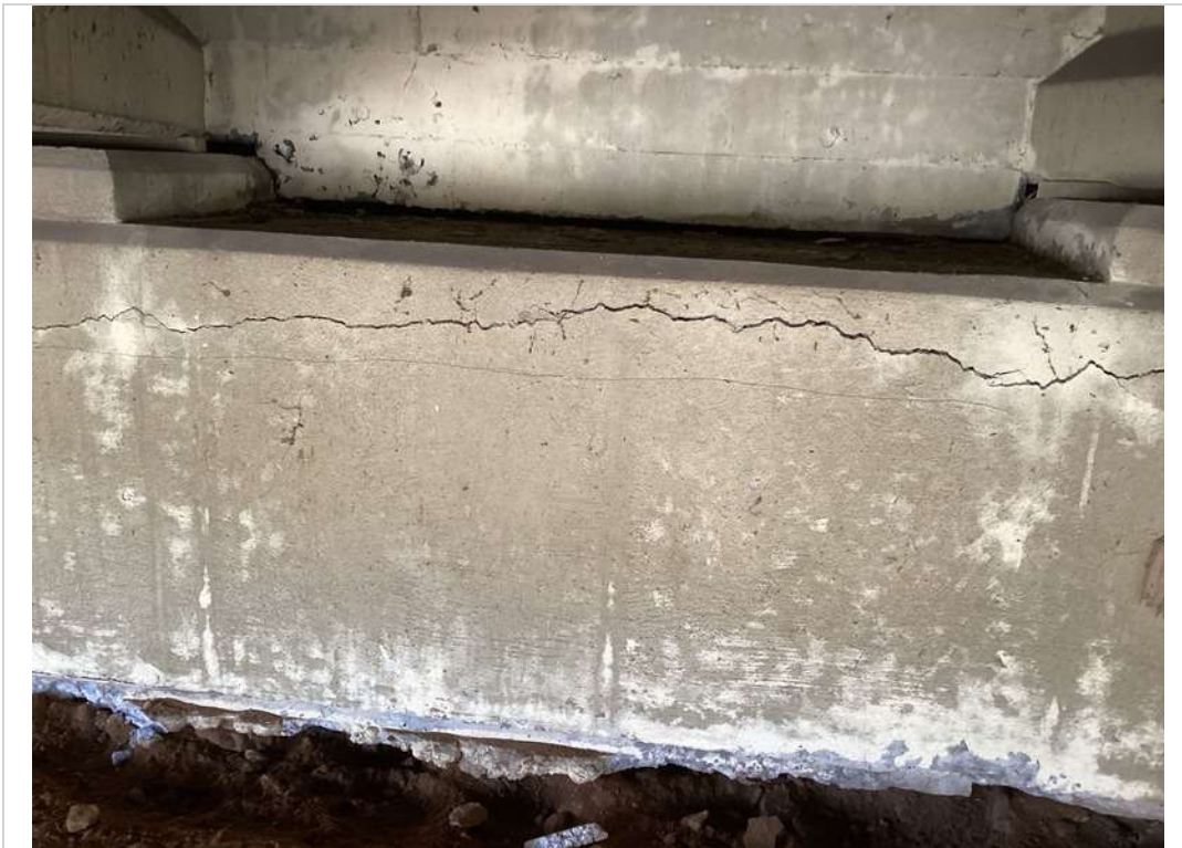
Abutment 1 delam on cap under Bay C
