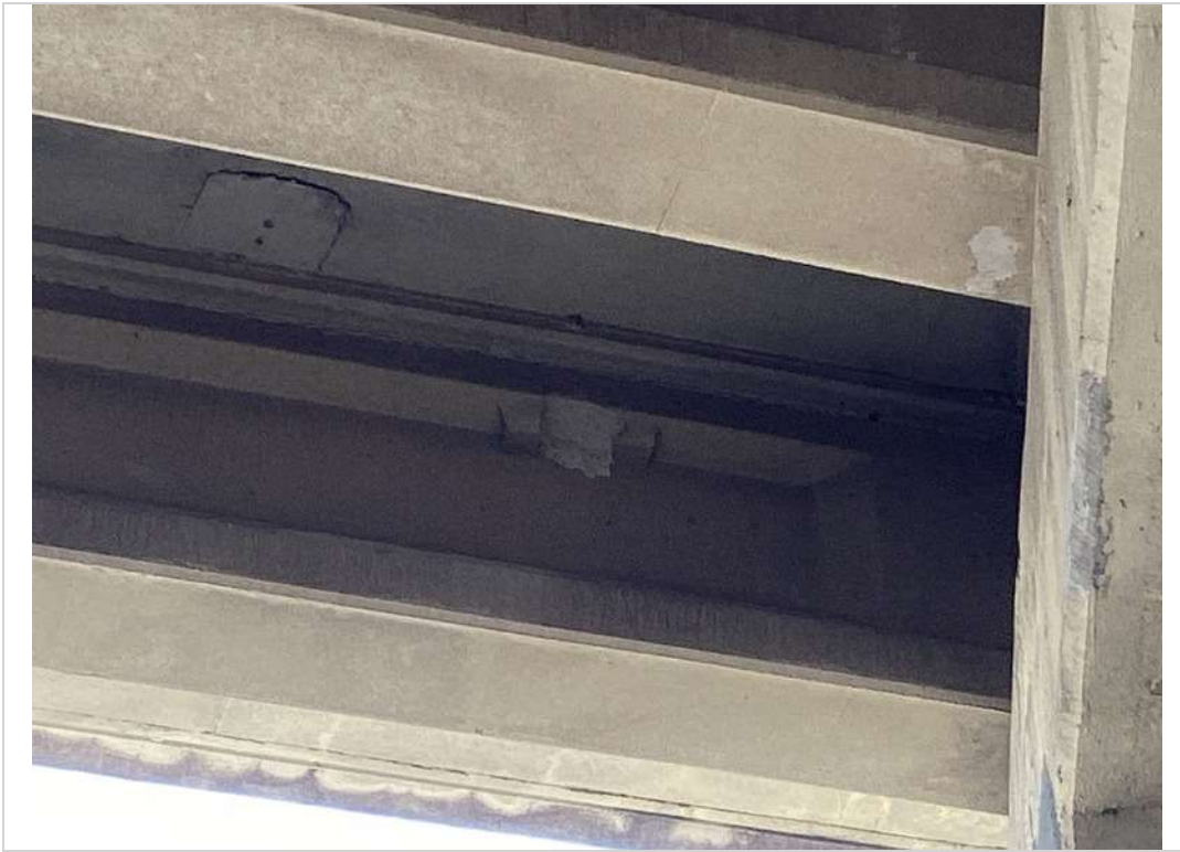
Span 3 delam in top flg left side of Beam F
