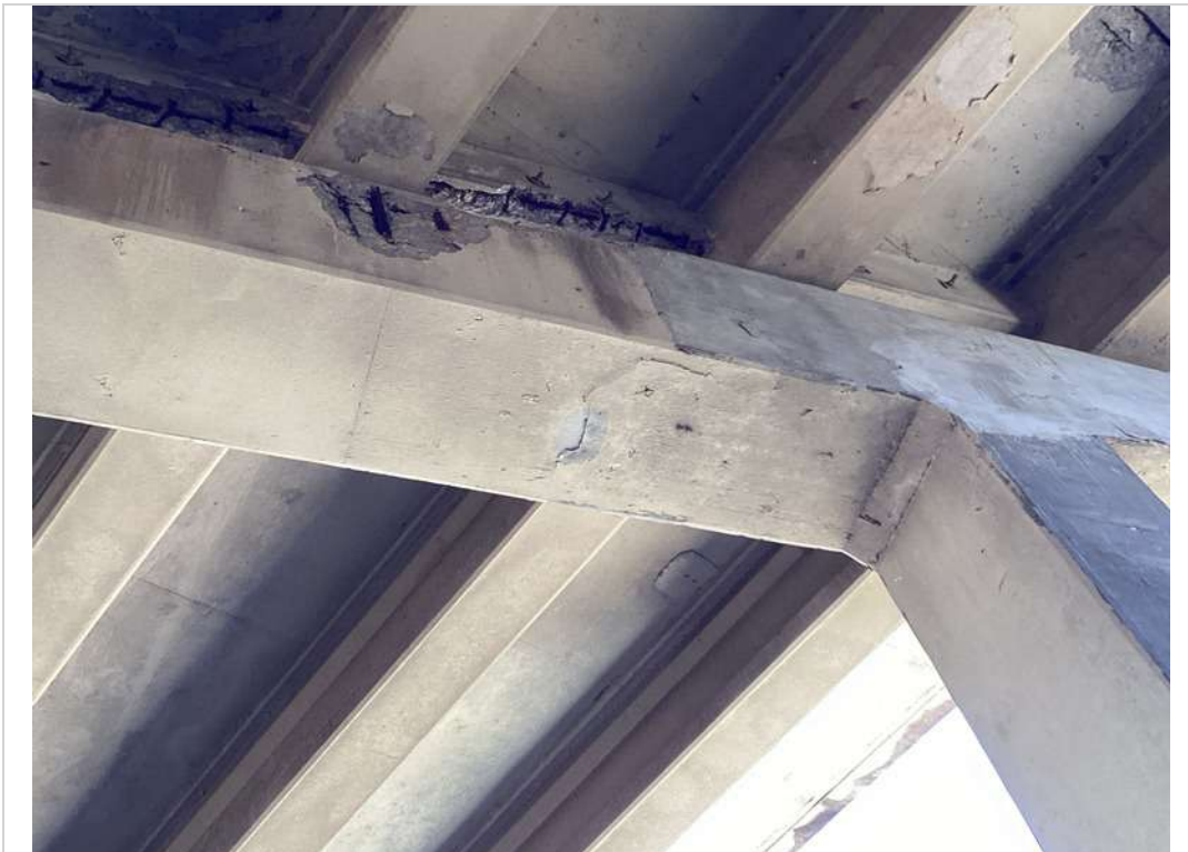
Bent 2 delam in bottom of cap
