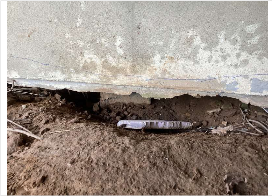
Abutment 1 undermining of cap w/ exposed pile w/ laminar corrosion under Bay E
