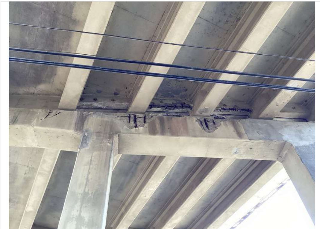
Span 2 spalling w/ exposed rebar in forward diaphragms
