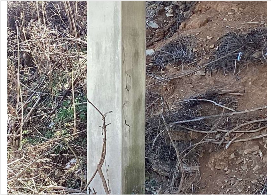
Bent 1 delam in Column C
