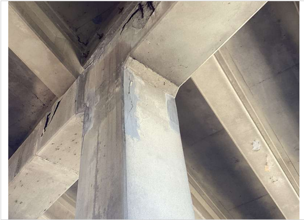
Bent 2 delam in right face of Column B
