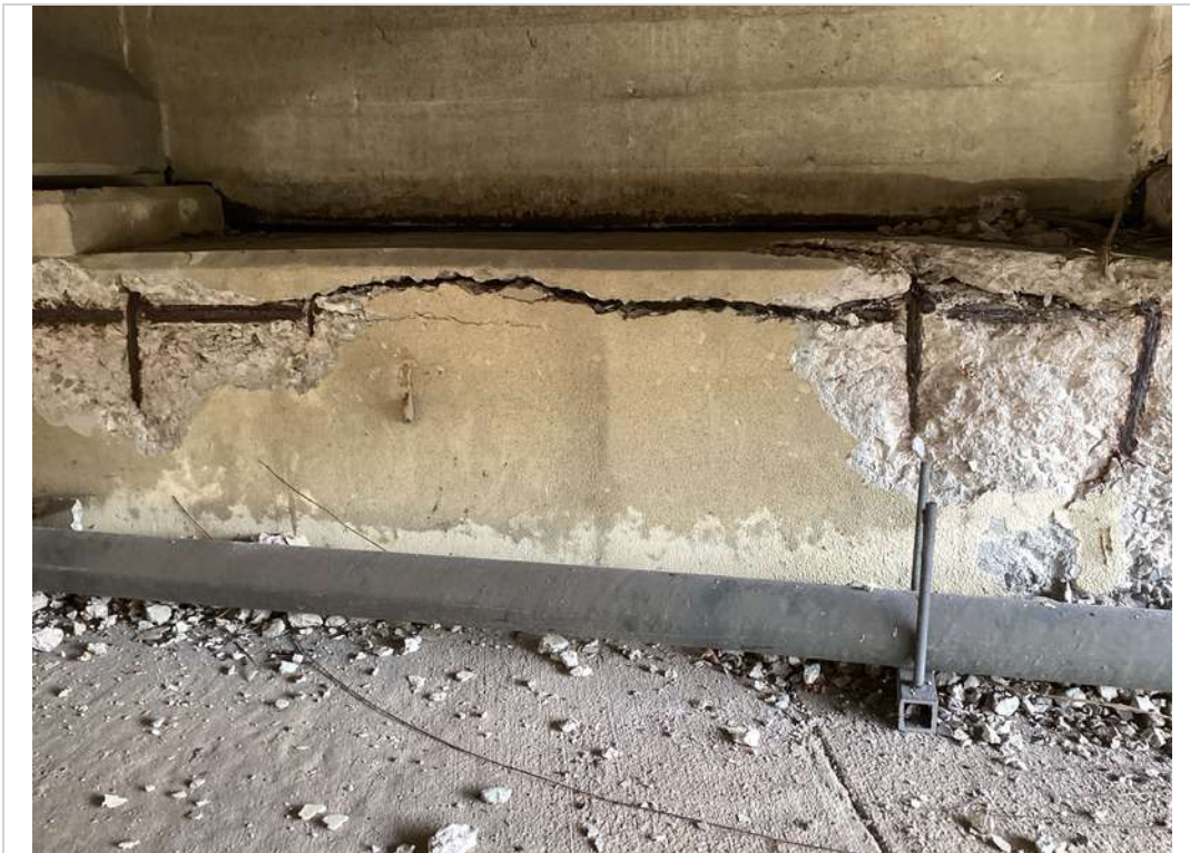
Abutment 2 spalling w/ exposed rebar and delam of top of cap under Bay D
