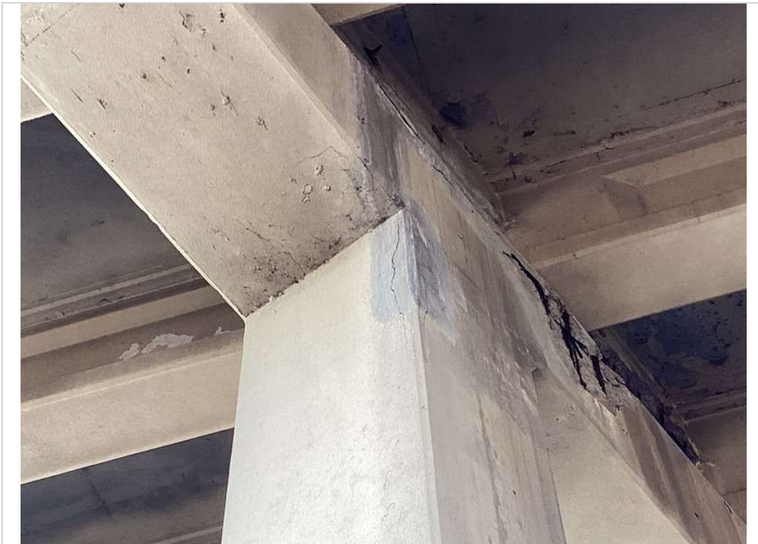
Bent 2 delam in front and left faces of Column B
