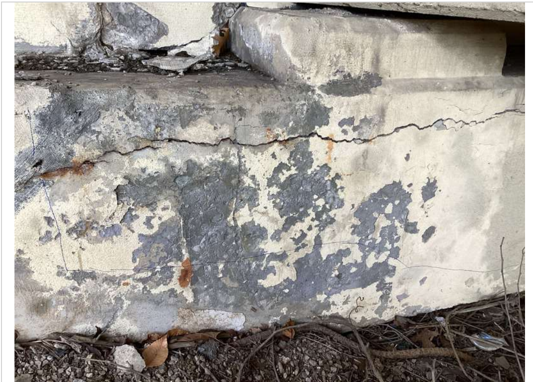
Abutment 1 delam on cap under right overhang
