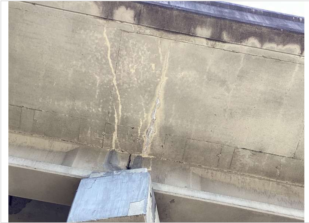
Spans 2 and 3 HL cracks w/ eff in right overhang over Bent 2
