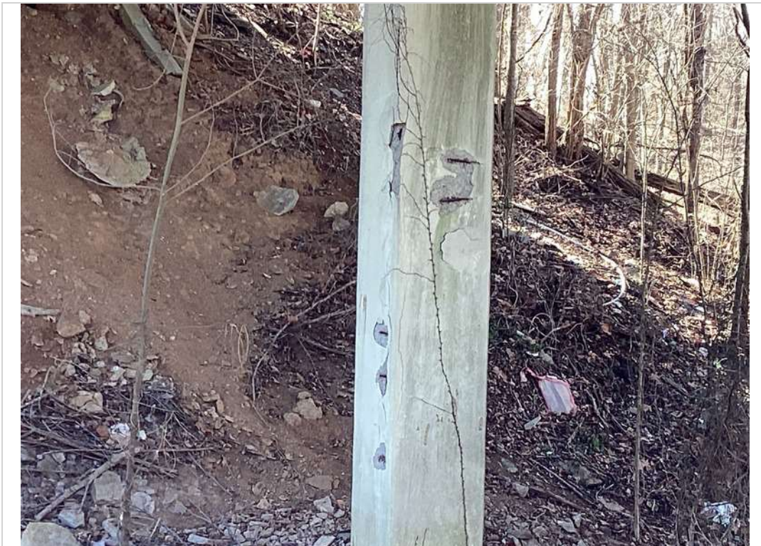
Bent 1 spalls w/ exposed rebar on right face of Column B
