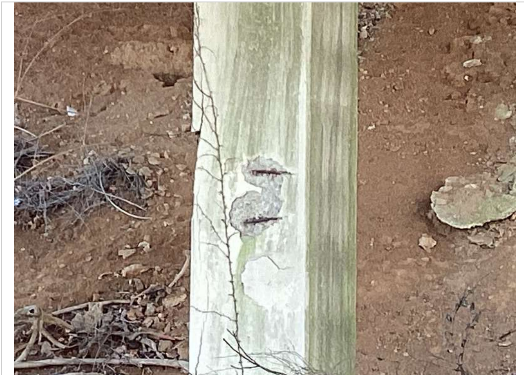
Bent 1 spall w/ exp. rebar on Column B
