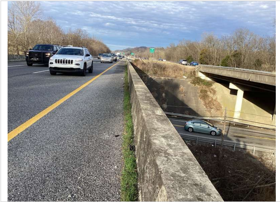
Vegetation growth along right parapet entire bridge length
