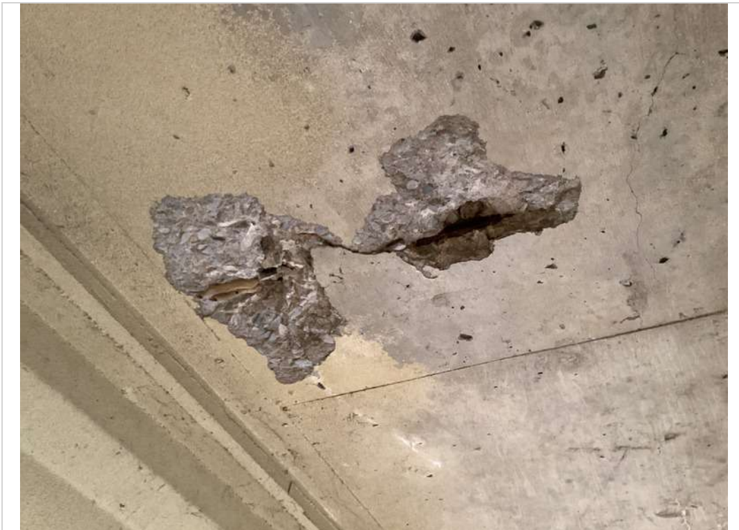
Span 1 spall w/ exposed rebar in Bay C
