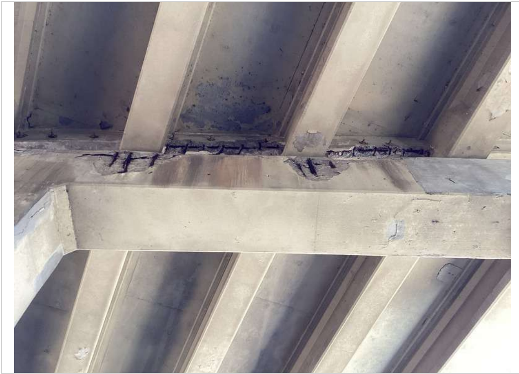
Bent 2 spalls w/ exposed rebar in front face of cap
