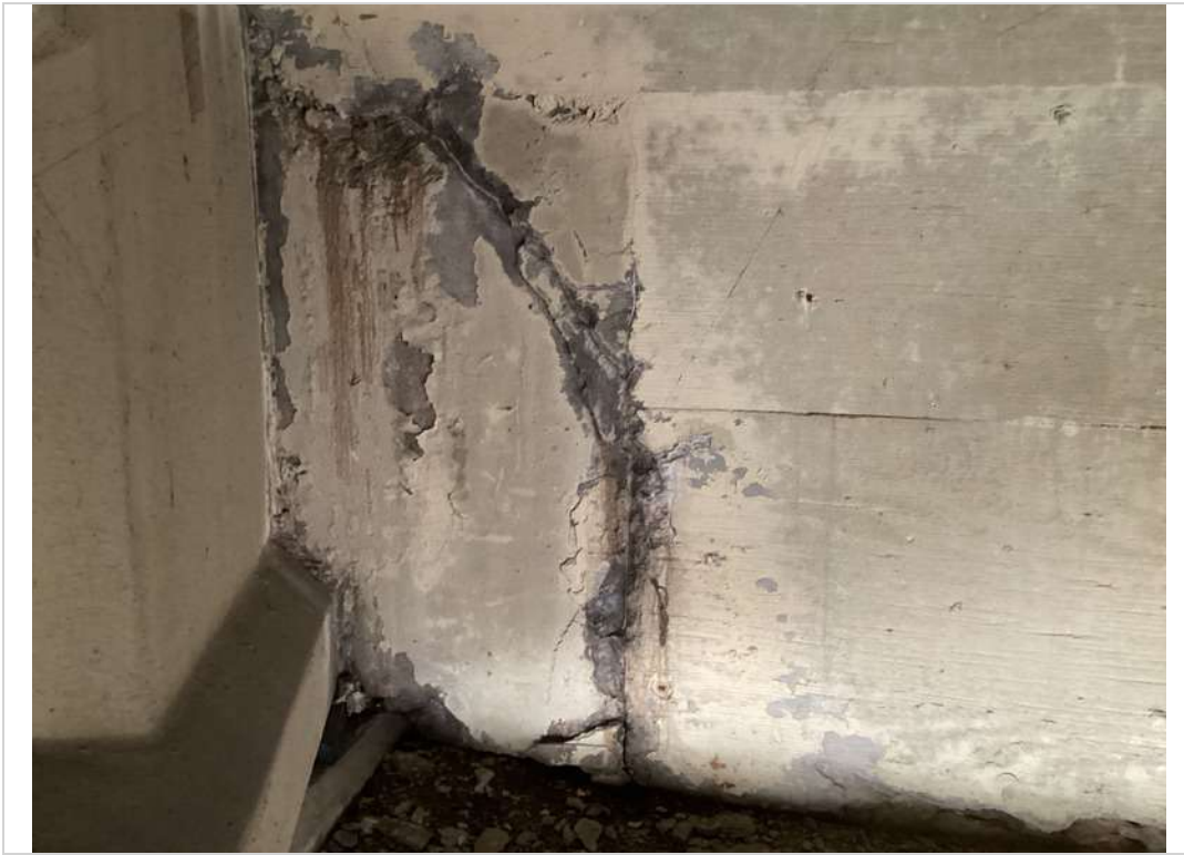
Abutment 1 crack and spalls along construct. joint under Bay A
