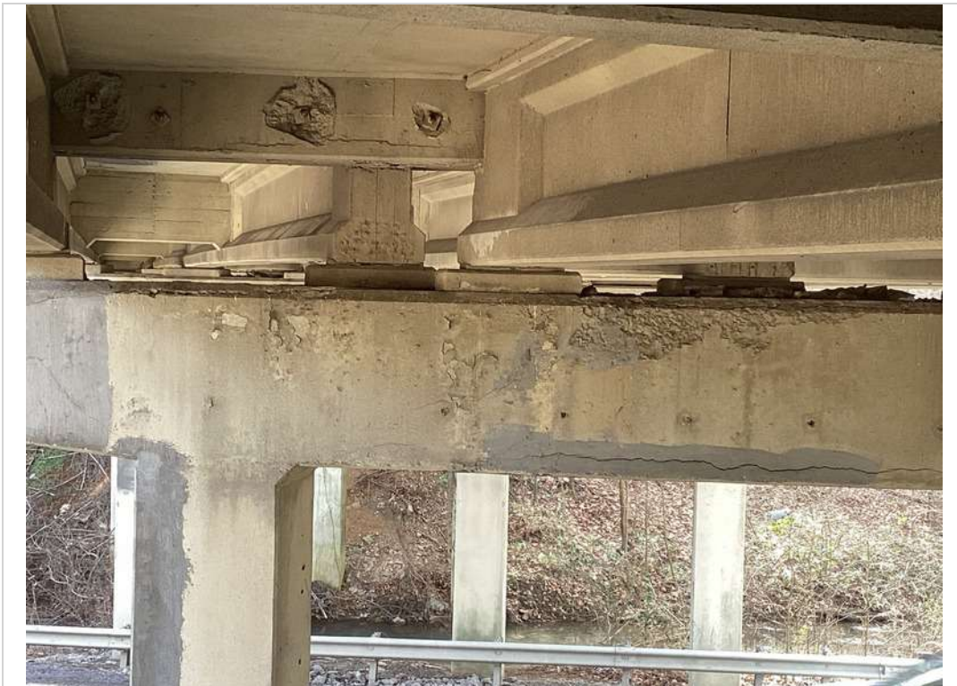
Bent 3 delams along top of cap between Beams C and E of Span 4
