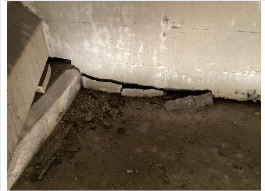
Abutment 1 spall on backwall under Bay D
