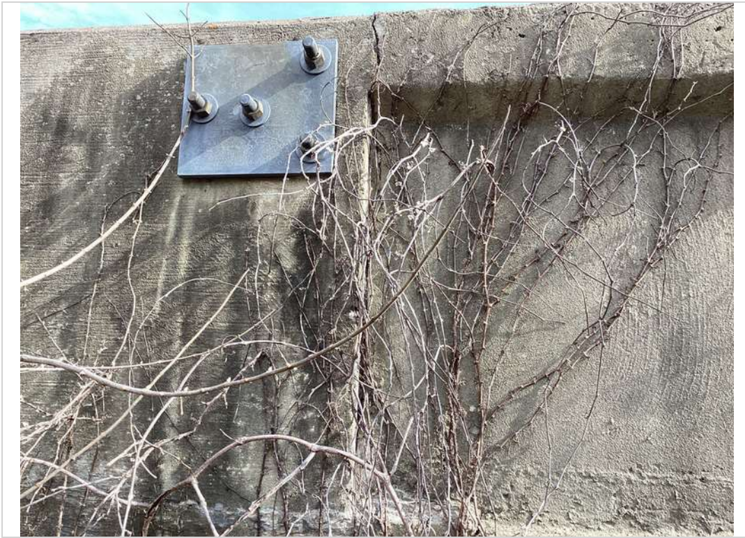
Abutment 2 1/16" crack in parapet over left wingwall
