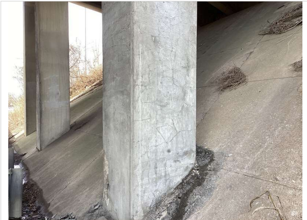
Bent 3 HL map cracking w/ iso 1/32" cracks in right face of Column C
