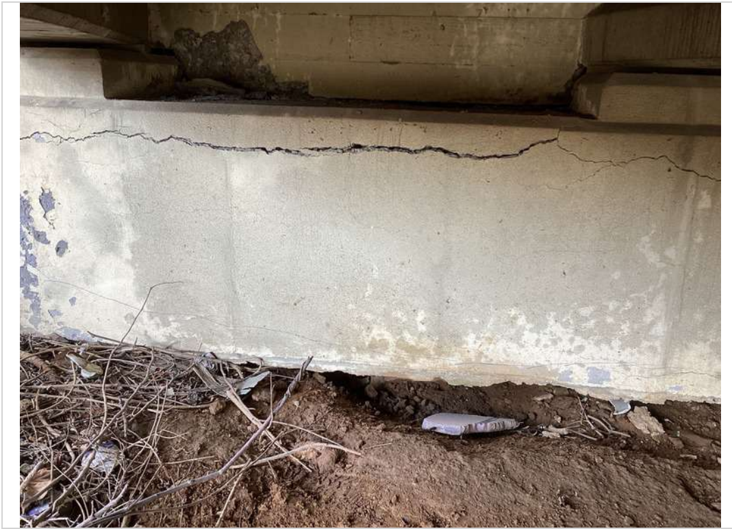
Abutment 1 delam on cap under Bay E
