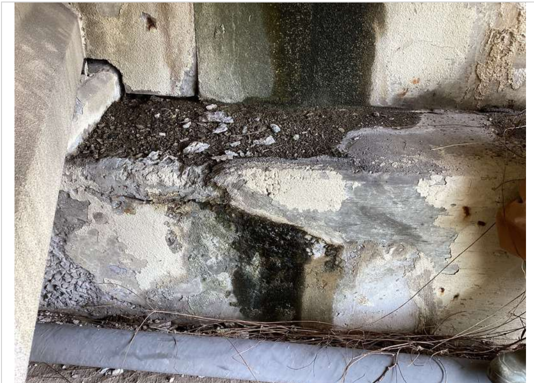
Abutment 2 spalling on top of cap under right overhang
