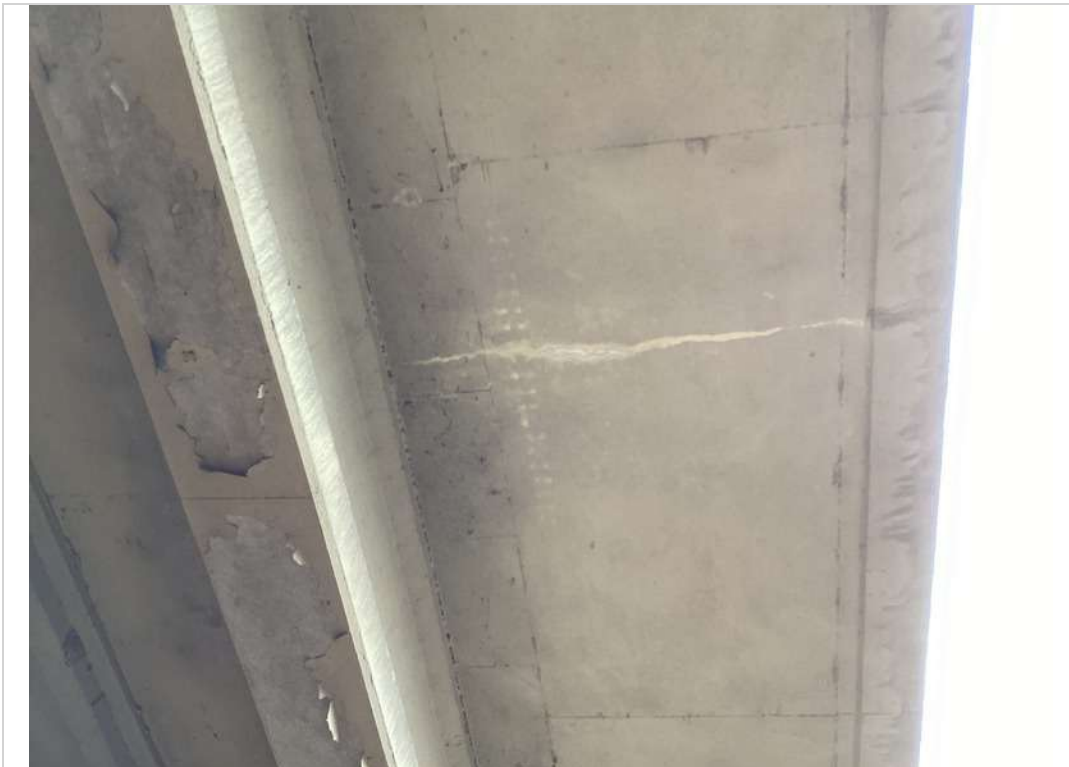
Span 1 crack w/ eff in right overhang
