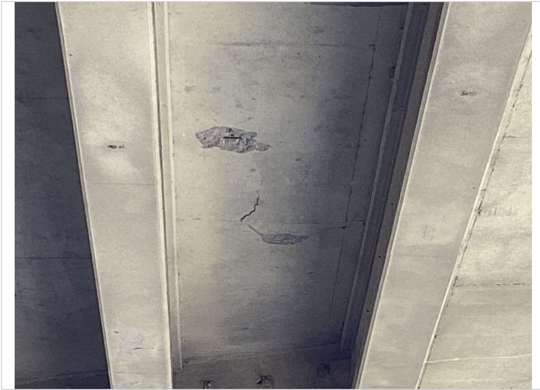
Span 3 delam and spall w/ exposed rebar in Bay E
