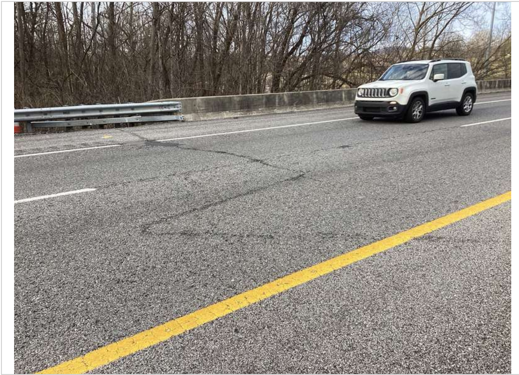
Wide crack and patch at beginning of bridge
