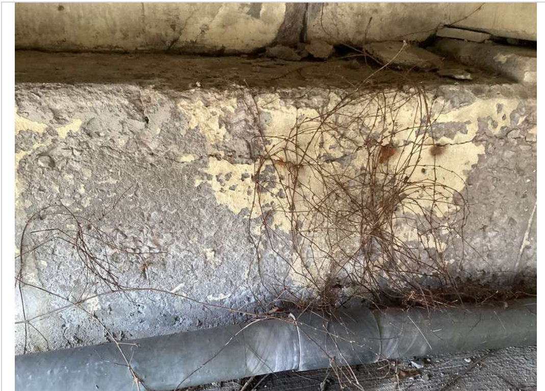
Abutment 2 deep honeycombing and 1/16" crack on cap under Bay A
