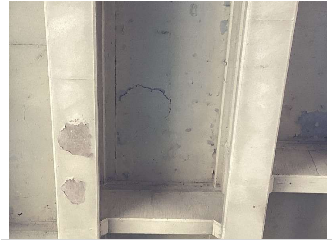
Span 2 delam in Bay C
