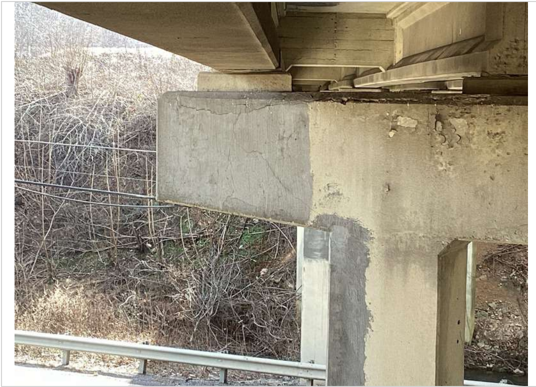
Bent 3 HL map cracking in back of cap to the right of Column C
