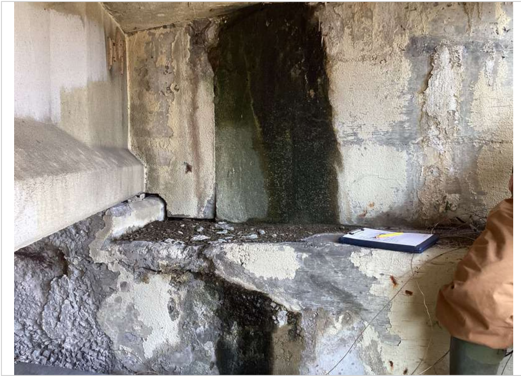
Abutment 2 water leakage and staining of backwall and cap under right overhang
