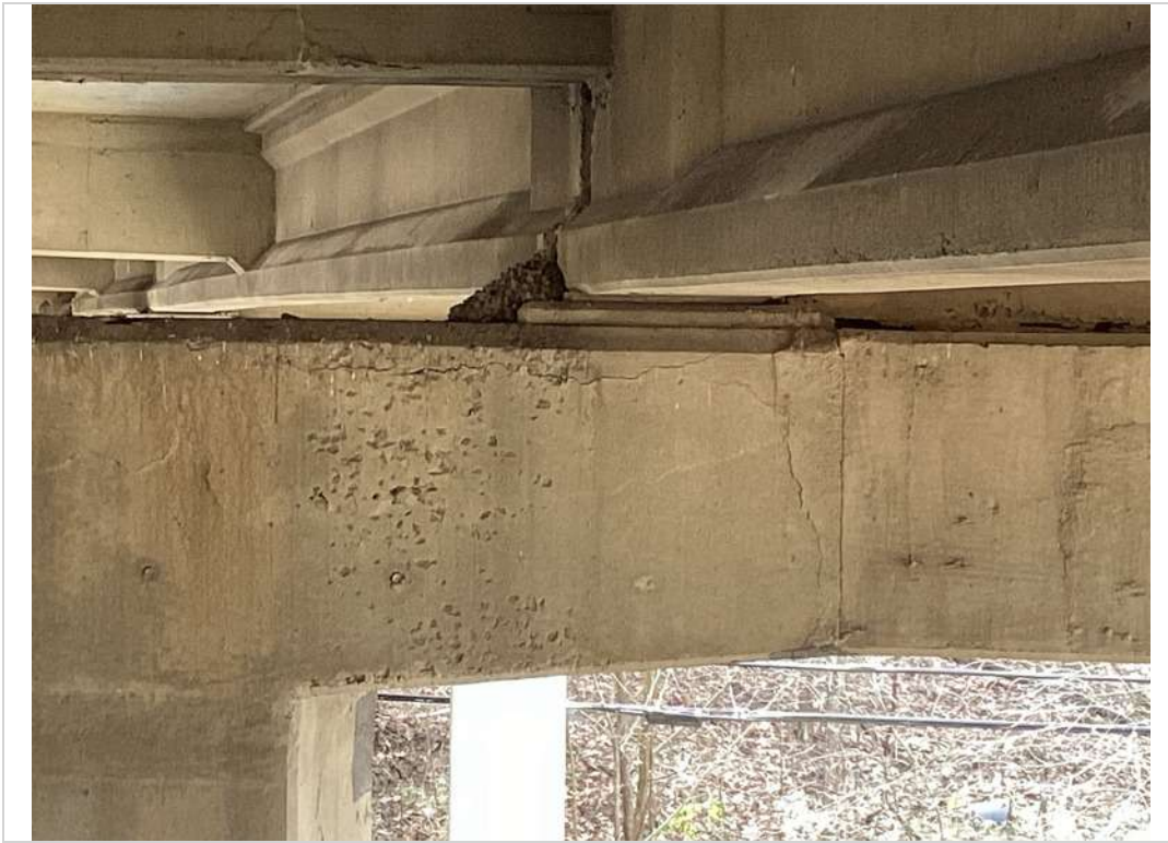
Bent 3 delam and HL crack in back of cap under Beam B
