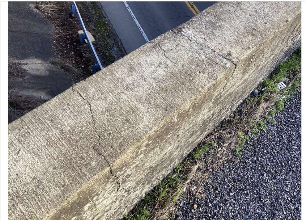
Span 4 moderate cracks in right parapet
