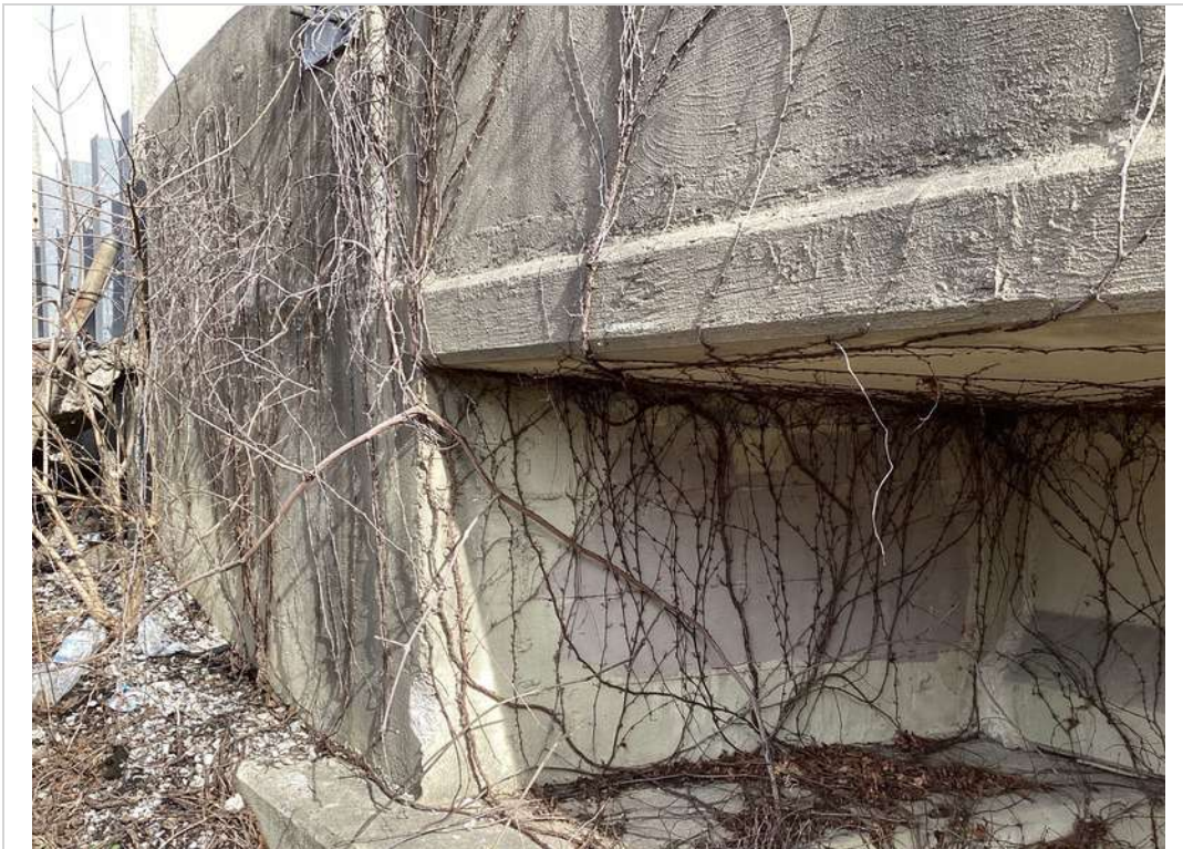
Abutment 2 vegetation growth on left wingwall and backwall
