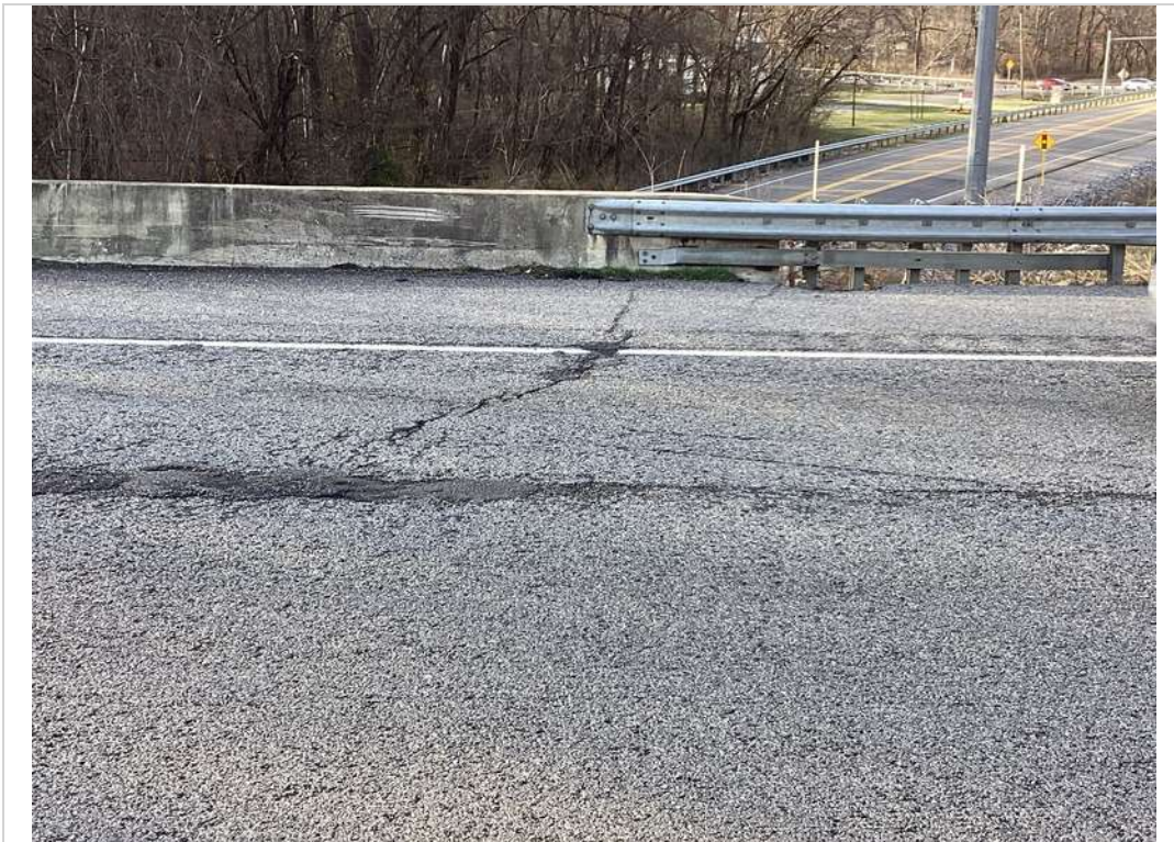
Wide crack in wearing surface at end of bridge
