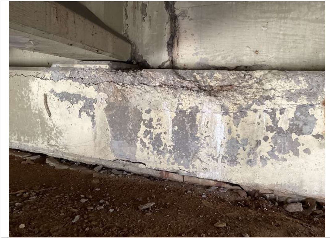
Abutment 1 whole face delam on cap under Beam B and delam and spall on cap under Bay A
