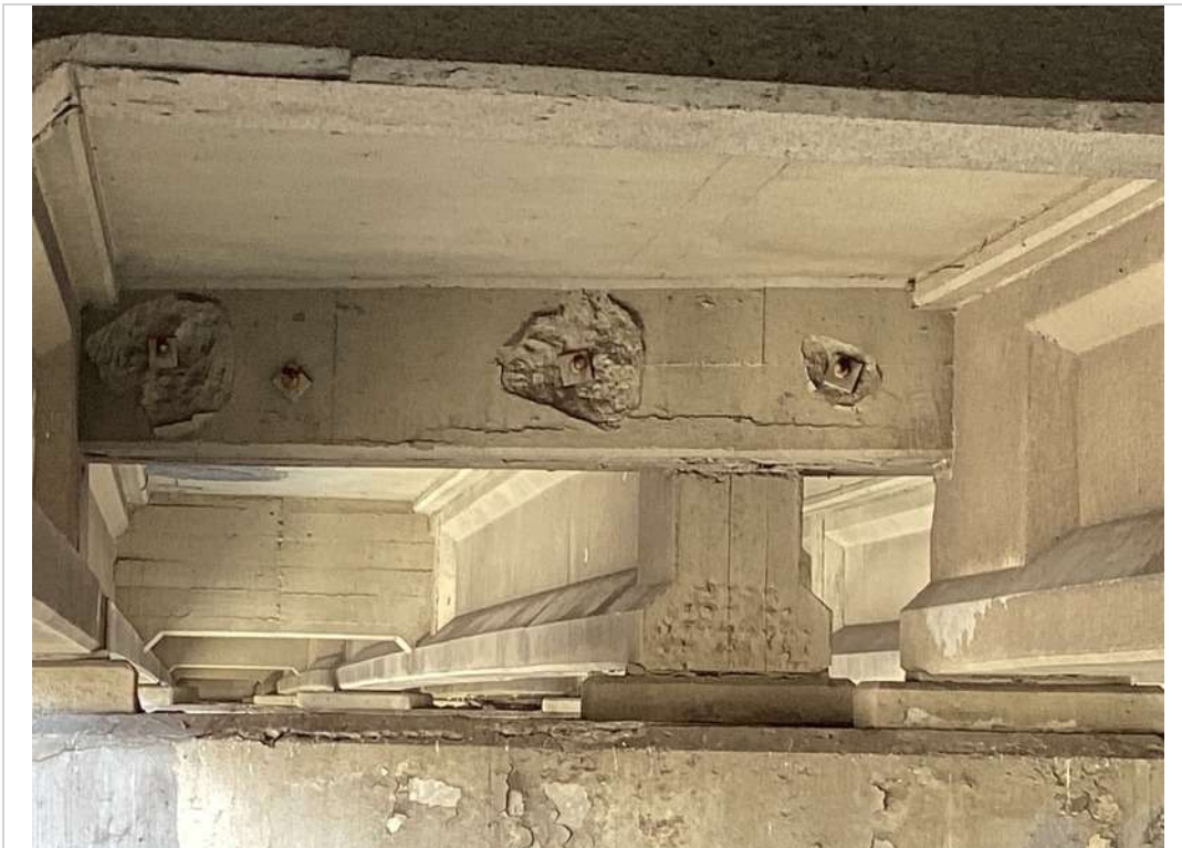
Span 4 delam and spalls in back diaphragms
