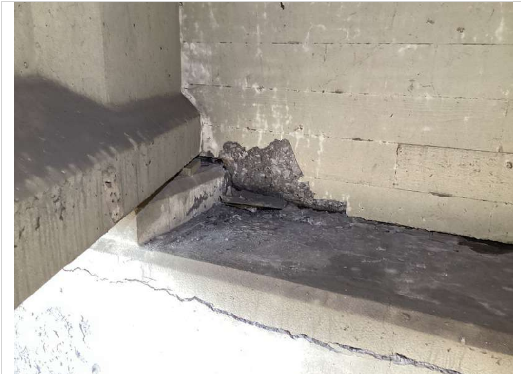
Abutment 1 spall on backwall under Bay E
