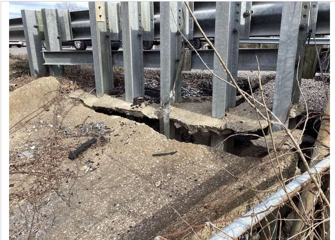
Abutment #2 failed left embankment drain
