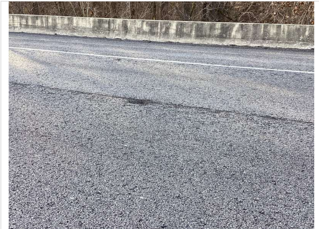
Span 2 pothole in wearing surface
