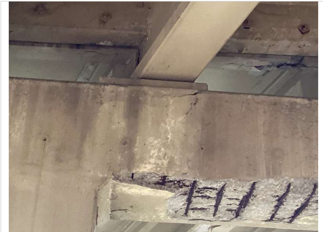
Bent 1 delam on front of cap under Beam C
