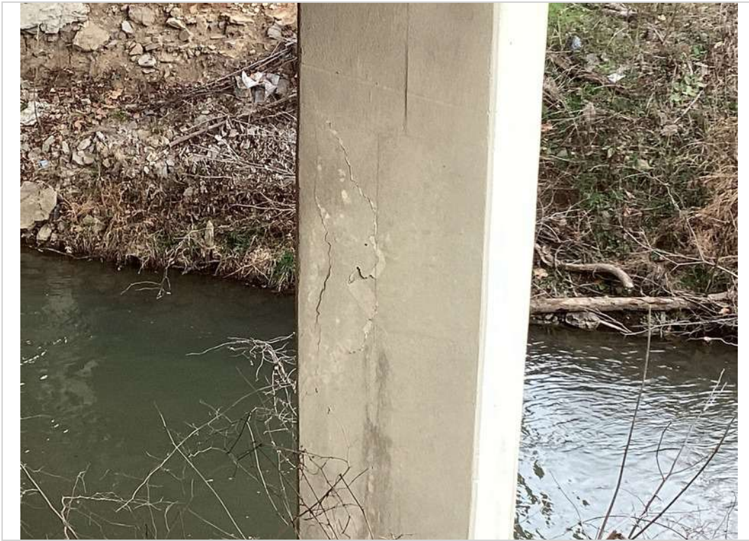
Bent 1 delam on front face of Column C
