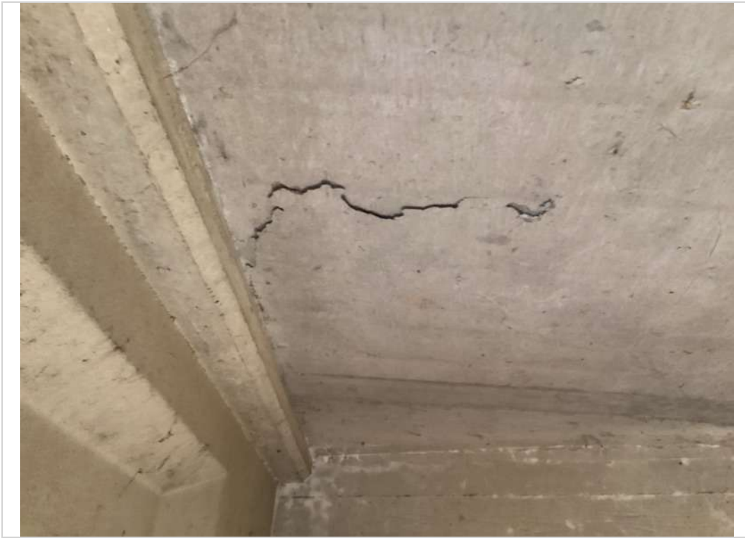
Span 1 delam in Bay E over Abutment 1
