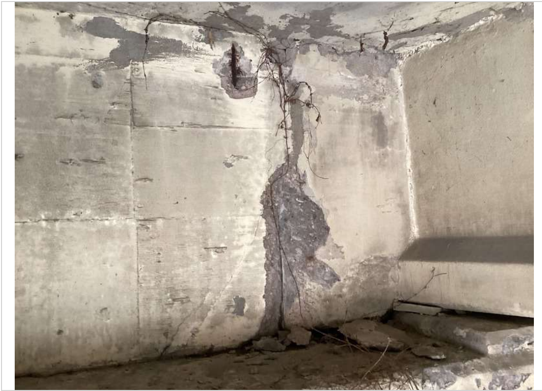
Abutment 2 spalls w/ exposed rebar in backwall of Bay A
