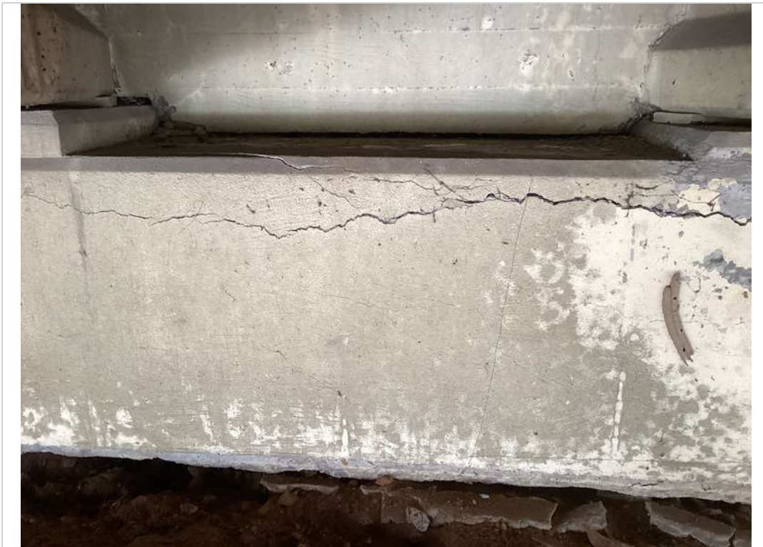
Abutment 1 delam on cap under Bay B
