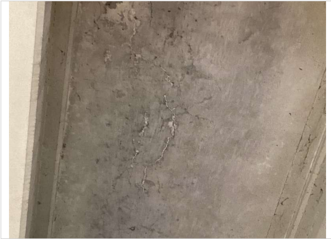
Span 1 HL cracks w/ eff in Bay C
