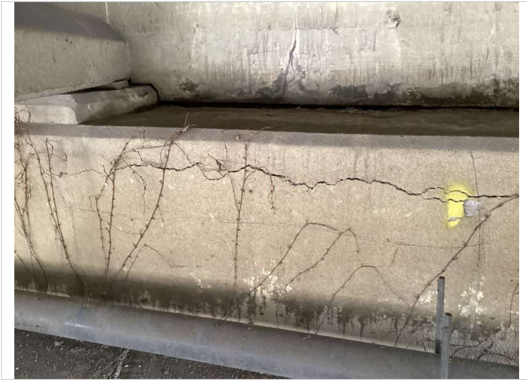
Abutment 2 delam on cap under Bay C
