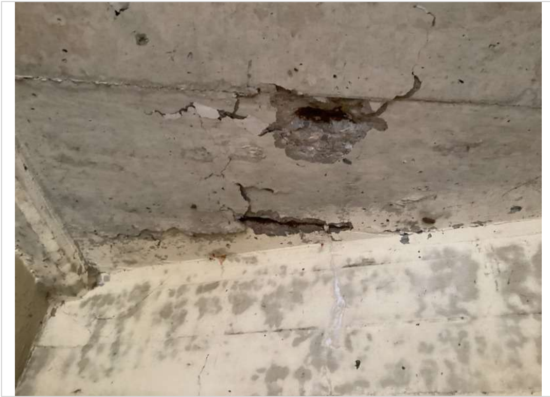
Span 1 spall w/ exposed rebar in Bay C over Abutment 1
