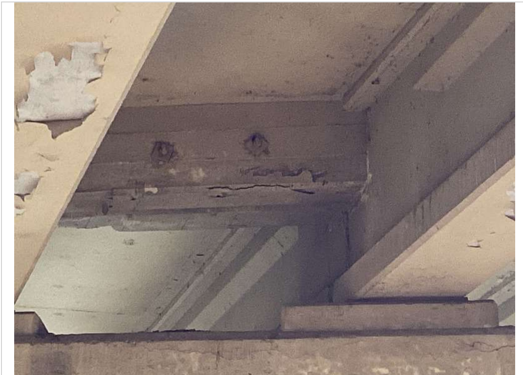
Span 1 delam in forward diaphragm
