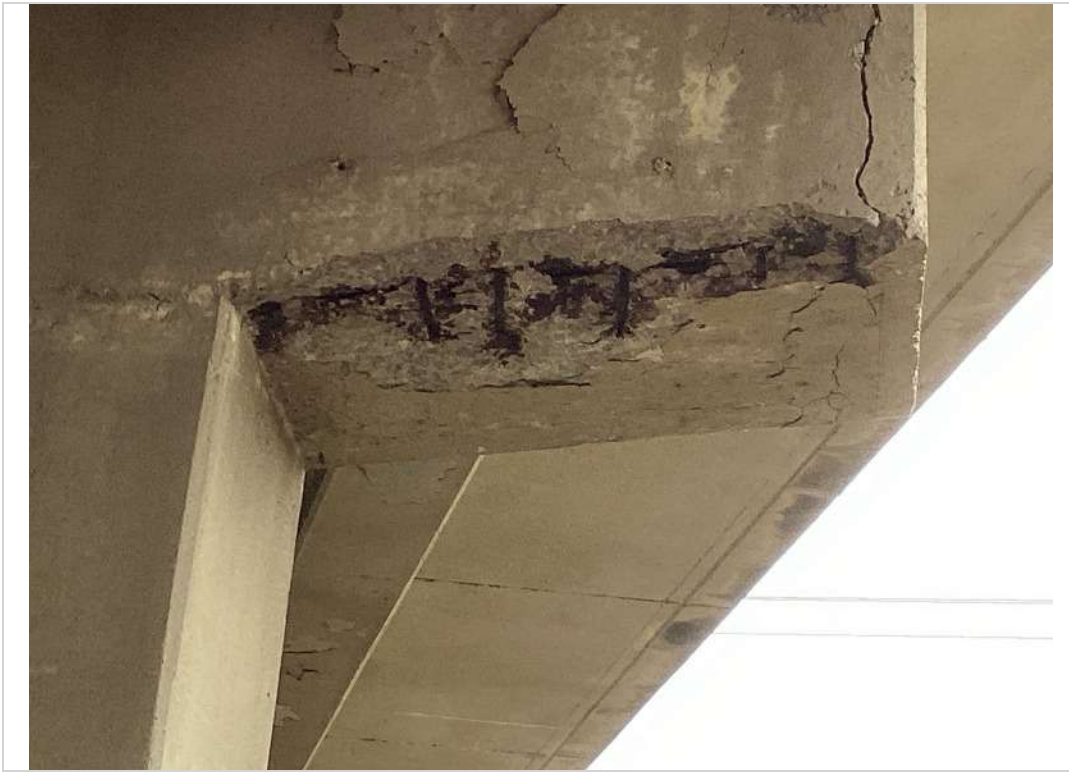
Bent 1 spall w/ exposed rebar on underside of cap to the right of Column C
