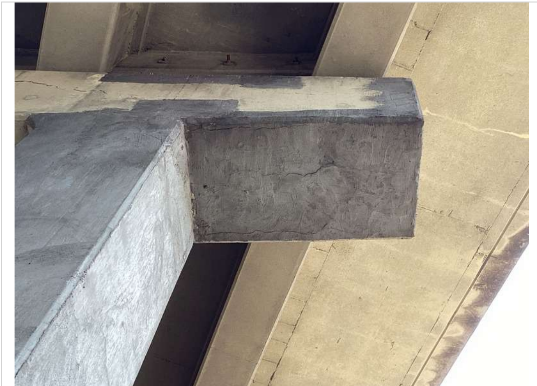
Bent 3 delam on underside of cap to the right of Column C
