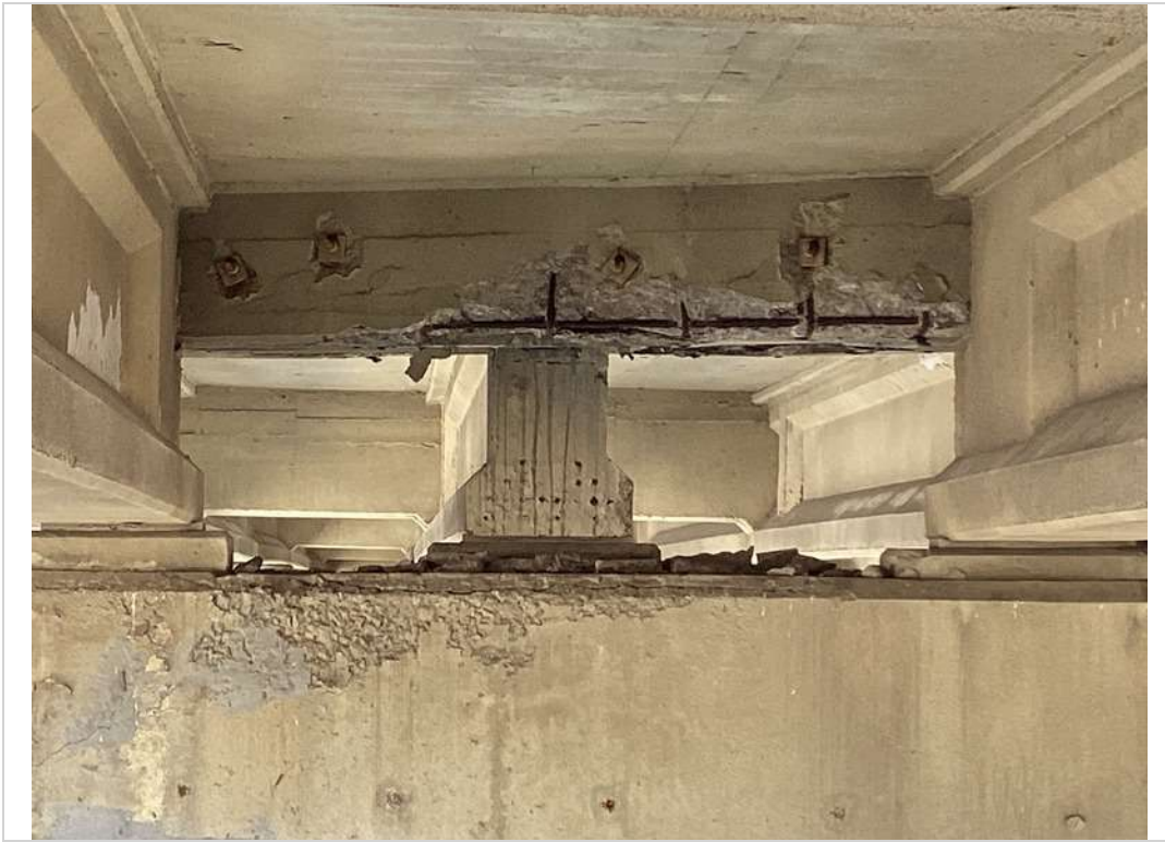
Span 4 spall w/ exposed rebar in back diaphragms
