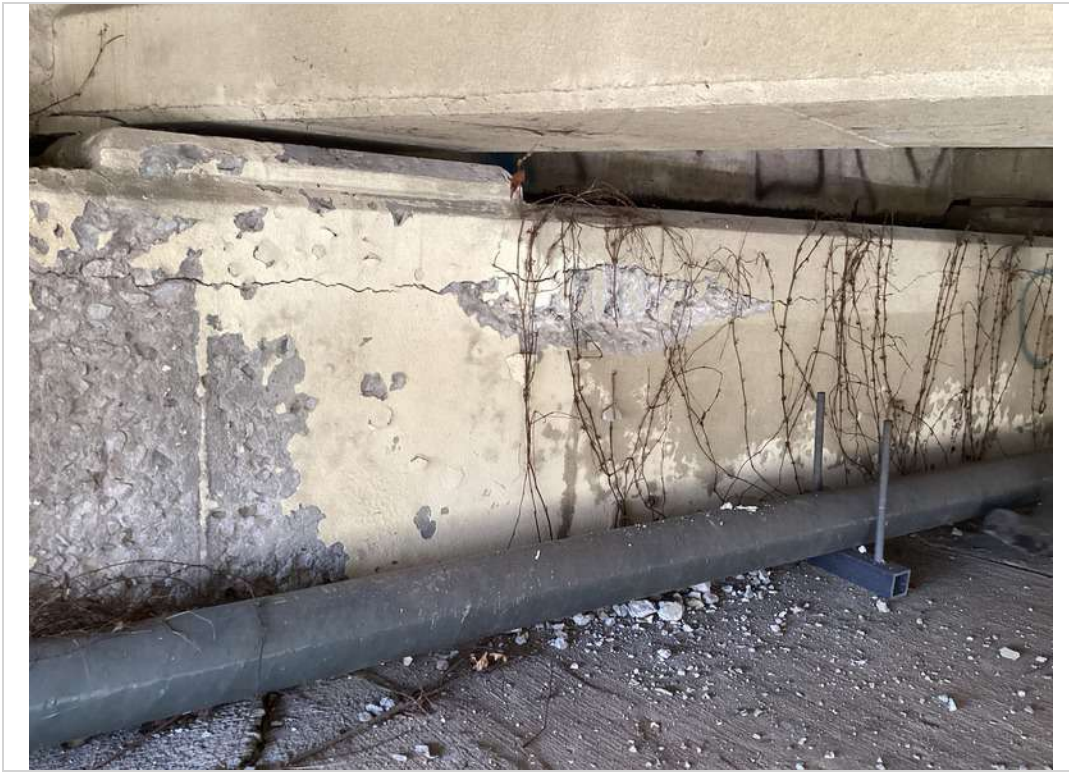
Abutment 2 spalling and wide crack on cap under Bay B
