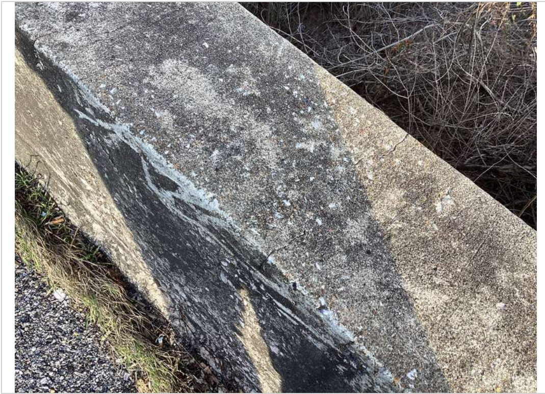
Typical HL crack in both parapets all spans
