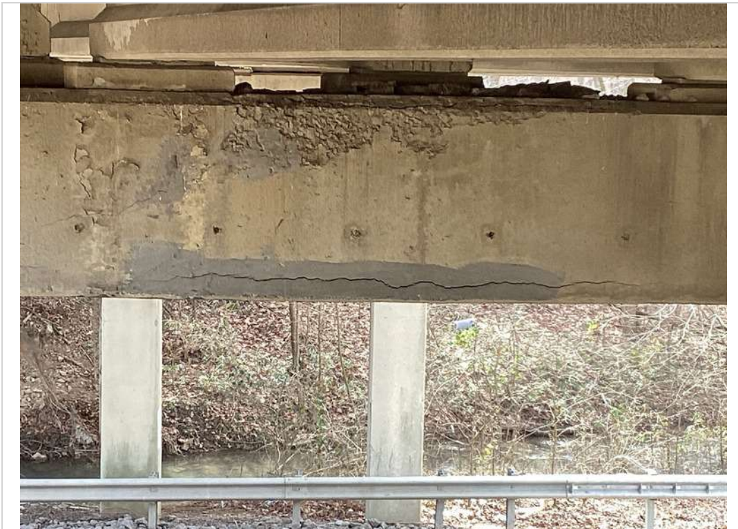
Bent 3 delam and honeycombing on back of cap between Columns B and C
