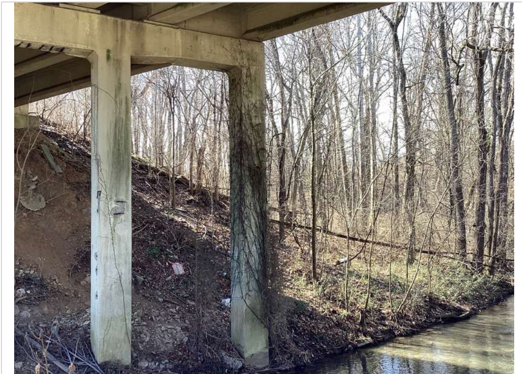
Bent 1 vegetation growth on Column A
