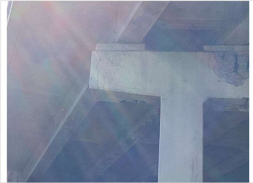
Bent 1 moderate cracks at right end and bottom of cap
