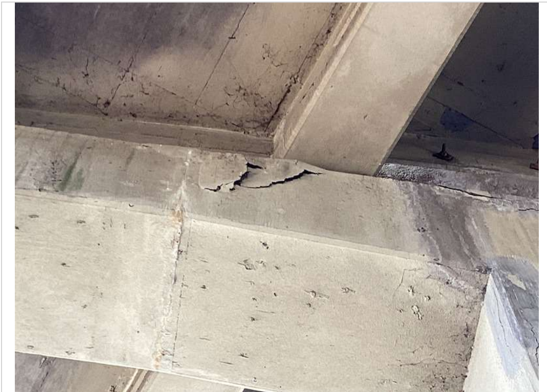
Bent 2 delam in front face of cap
