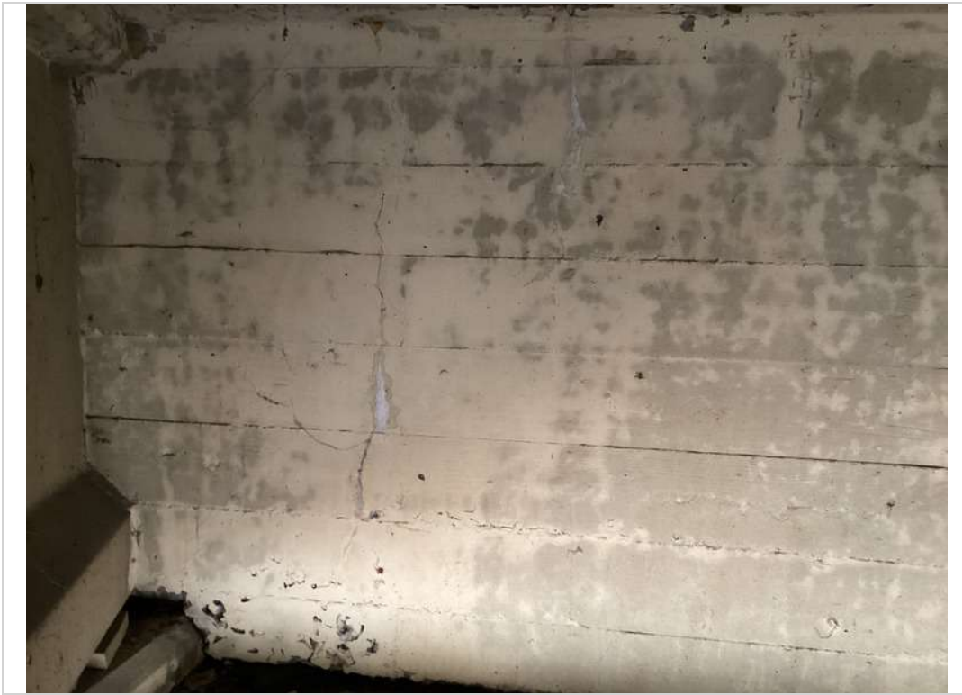
Abutment 1 HL cracks w/ eff on backwall under Bay C
