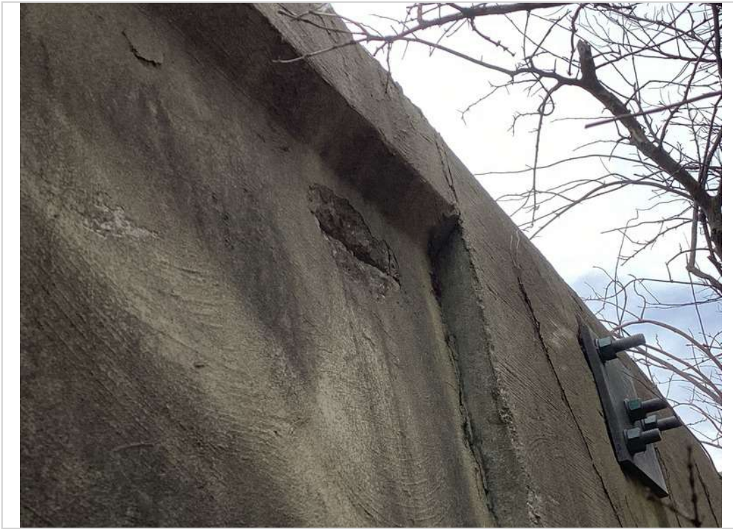
Span 1 spall w/ exposed rebar on left parapet over Abutment 1
