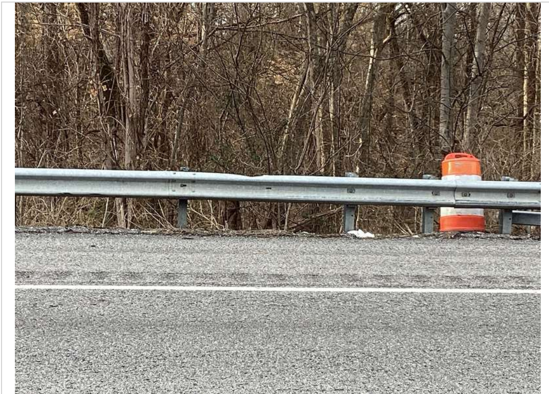
Approach 1 distortion in left side guardrail
