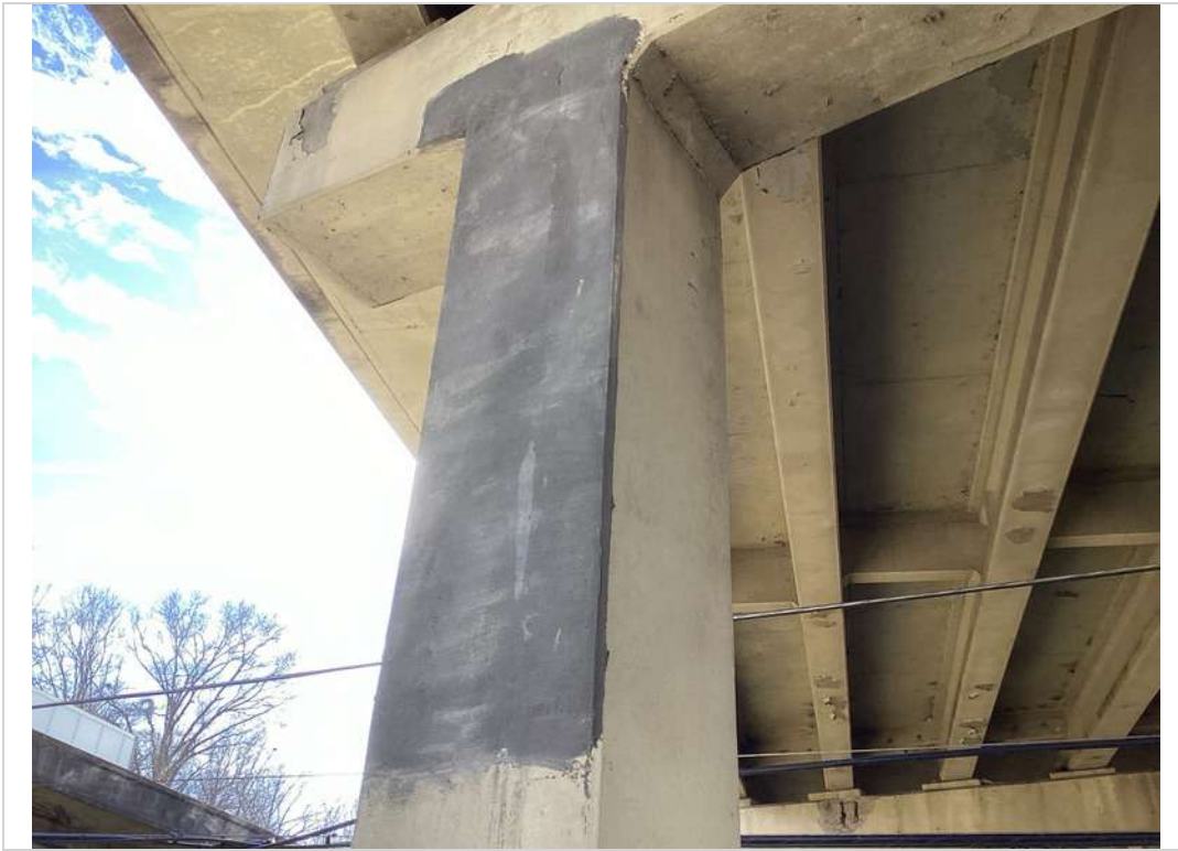
Bent 2 patch with HL cracks on back face of Column C
