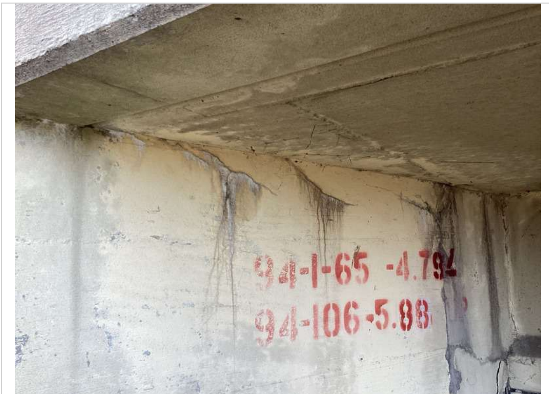
Abutment 1 cracks w/ hvly eff on backwall under right overhang
