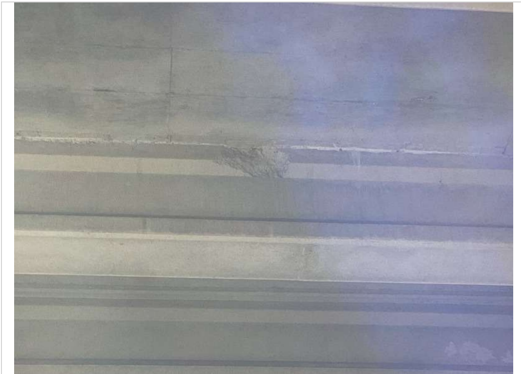
Span 3 spall in top flg left side of Beam B
