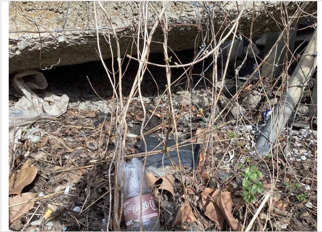
Abutment 2 undermining of left embankment drain
