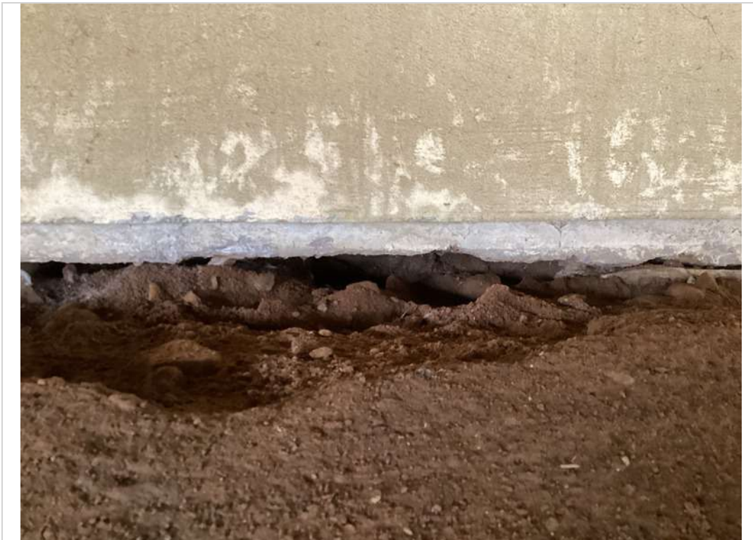
Abutment 1 undermining of cap under Beam C
