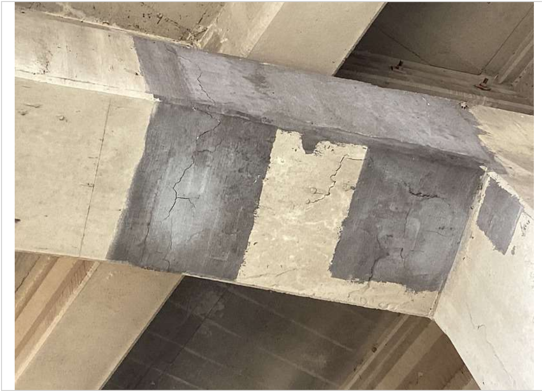
Bent 3 delam and moderate cracks on underside of cap between Columns A and B
