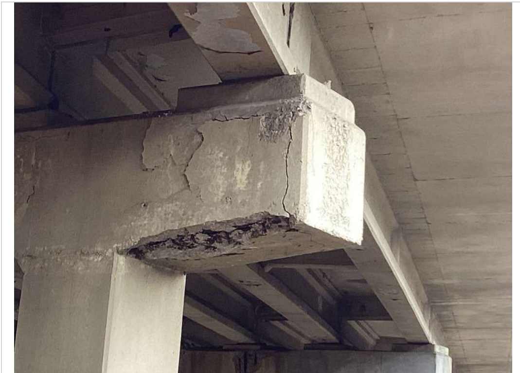
Bent 1 delam in cap front to the right of Column C
