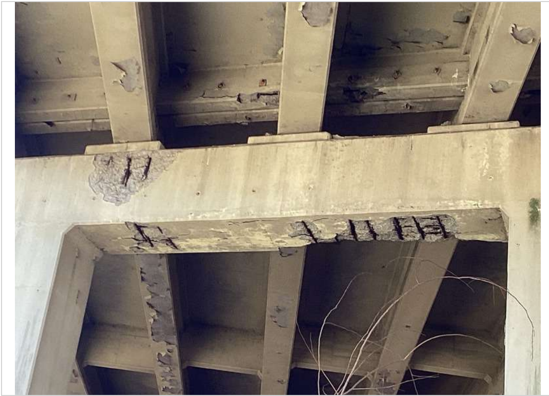
Bent 1 spalls w/ exp. rebar on back and bottom faces of cap
