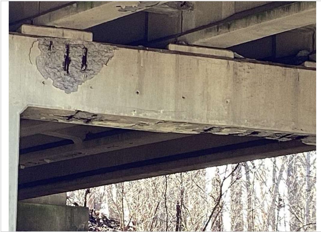
Bent 1 1/16" crack in back of cap
