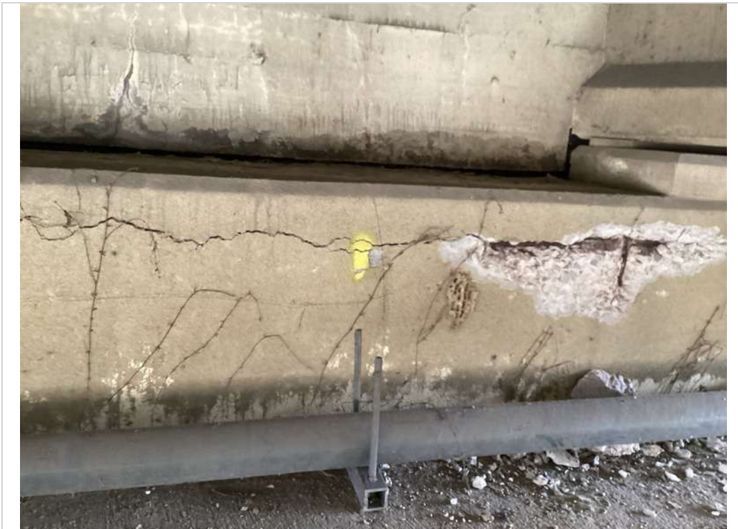
Abutment 2 spalling w/ exposed rebar and wide crack on cap under Bay C
