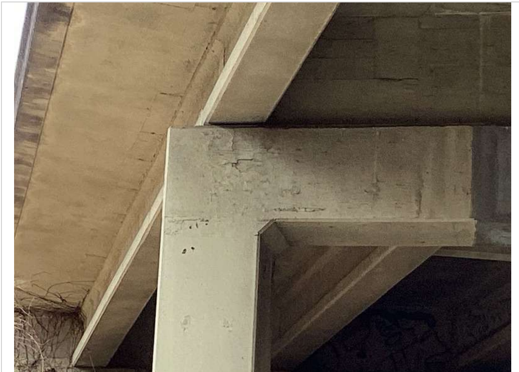
Bent 3 delam on front of cap over Column A
