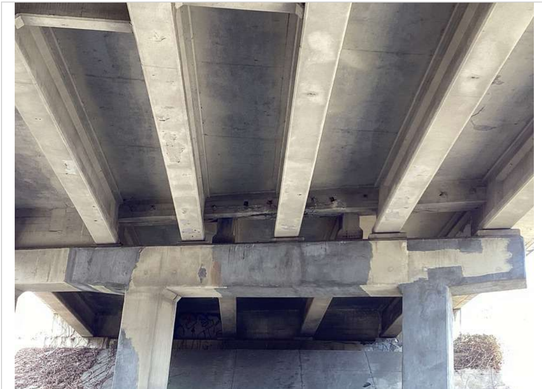
Span 3 mod cracks and delam in forward diaphragms
