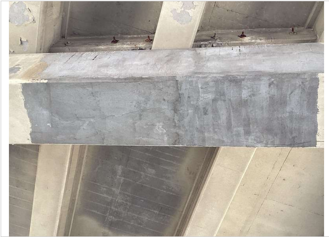
Bent 3 delam in patch on underside of cap between Columns B and C
