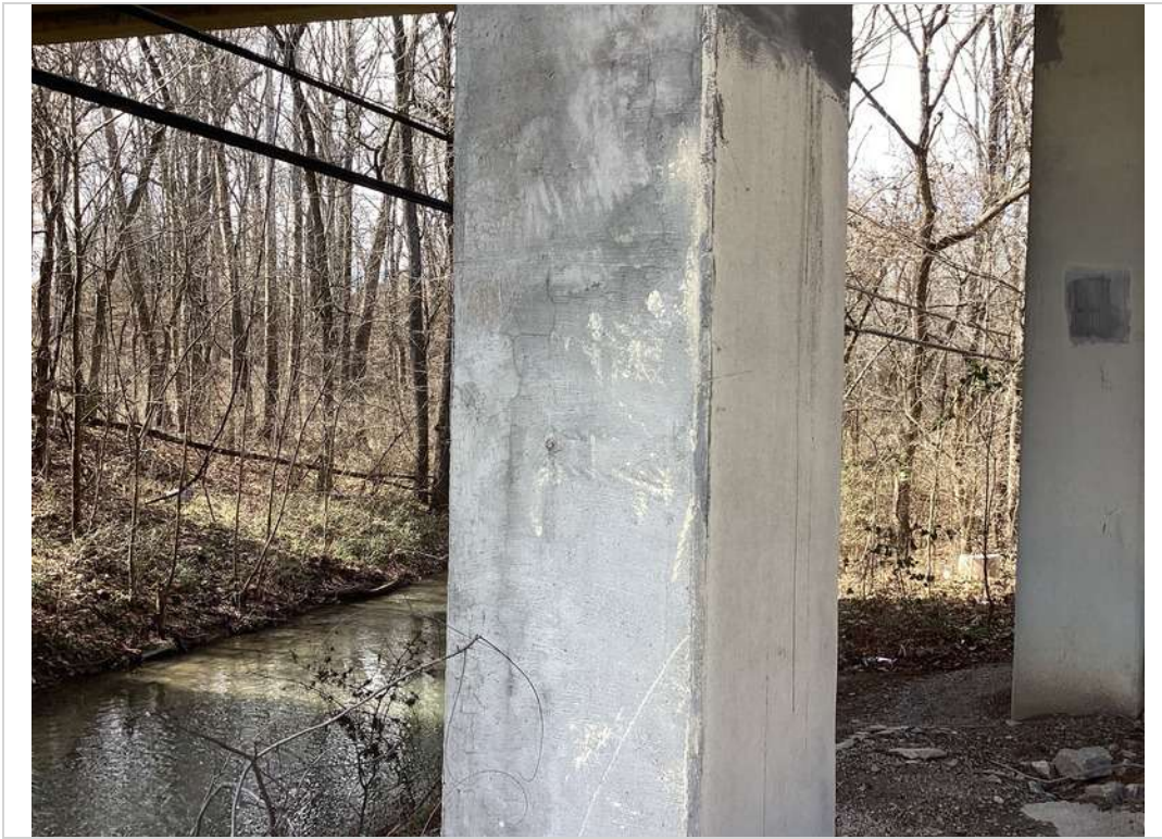
Bent 2 HL map cracking in right face of Column C
