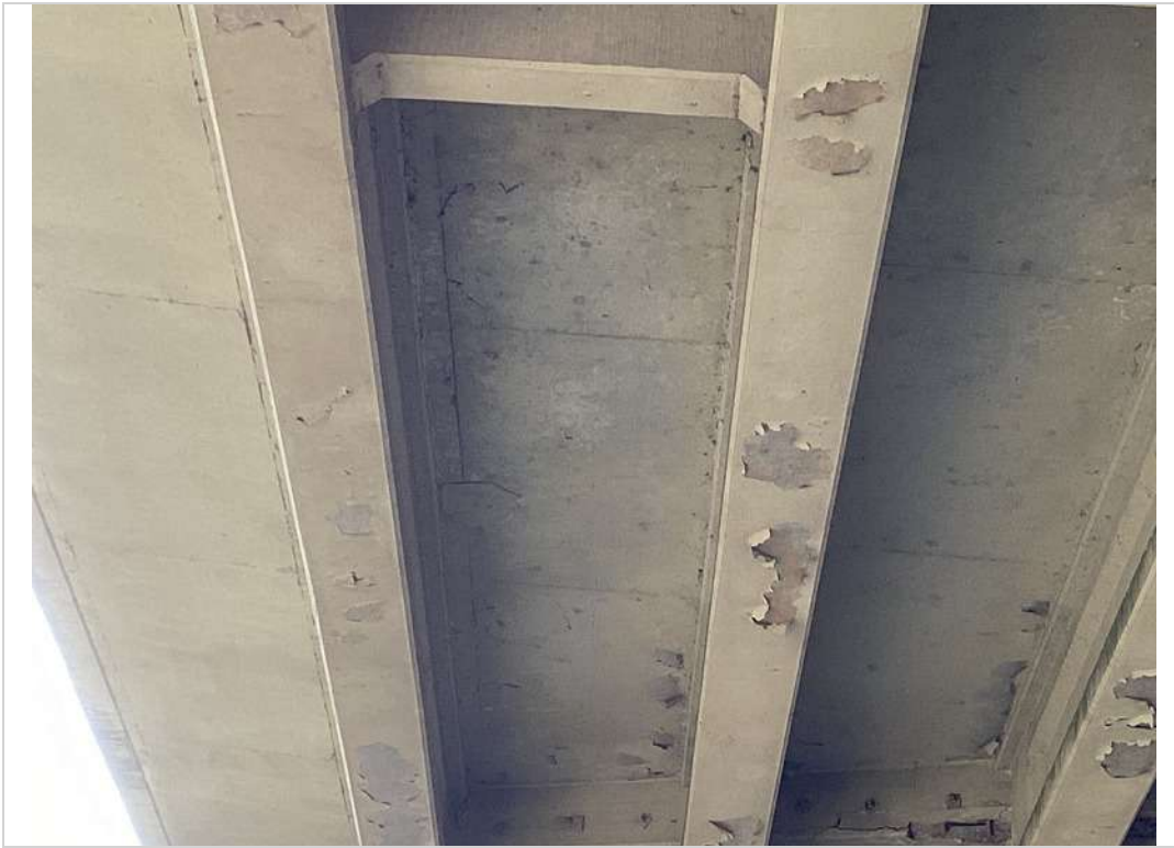
Span 2 delams in Bay E
