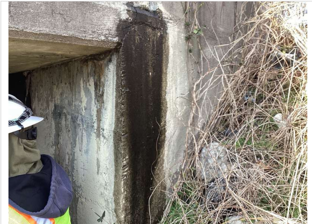
Abutment 2 1/16" crack w/ water leakage and staining in right wingwall
