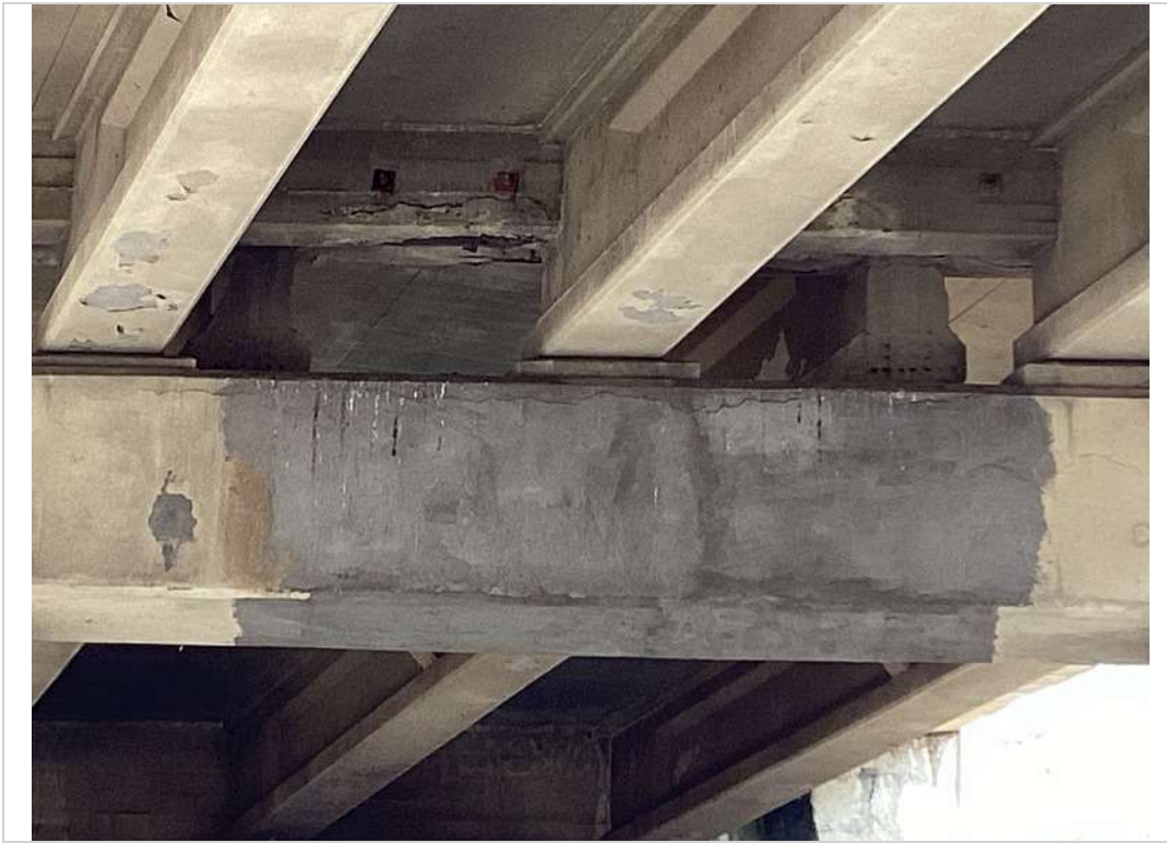
Bent 3 mod crack through patch on front of cap
