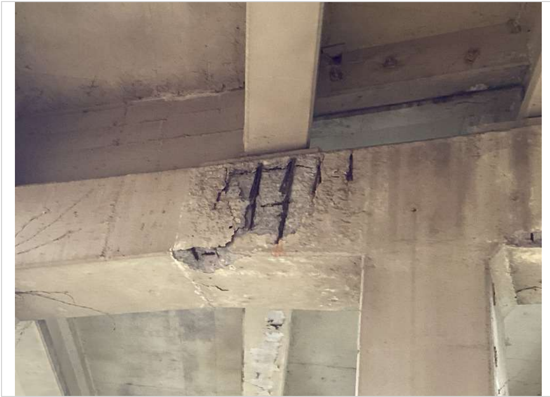
Bent 1 spall w/ exposed rebar on front of cap under Beam B
