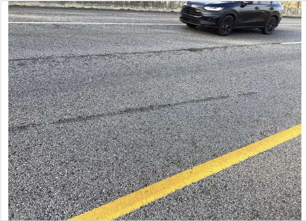
Span 2 gouge in wearing surface
