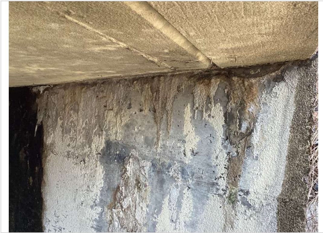
Abutment 2 heavy eff on backwall under right overhang
