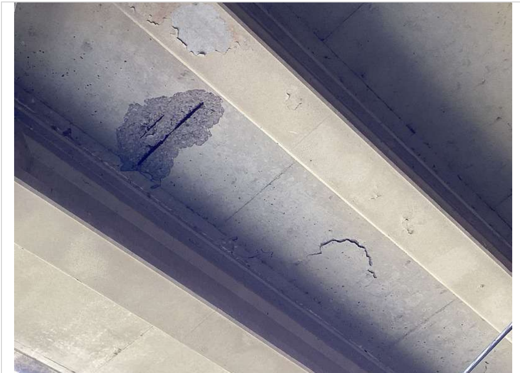
Span 2 delam and spall w/ exposed rebar in Bay E
