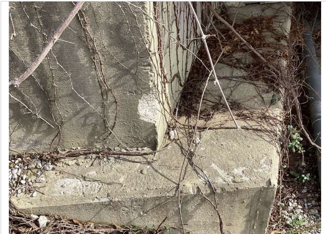
Abutment 2 spall on corner of left wingwall and backwall
