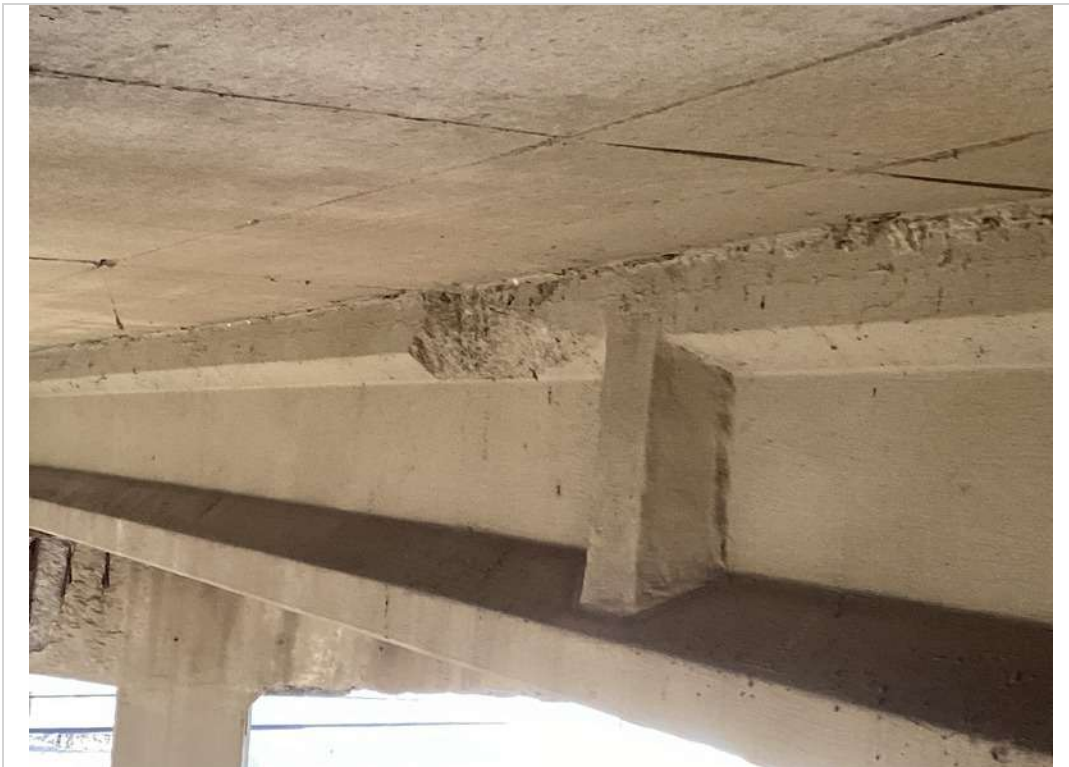
Span 1 spall on left side top flg of Beam B
