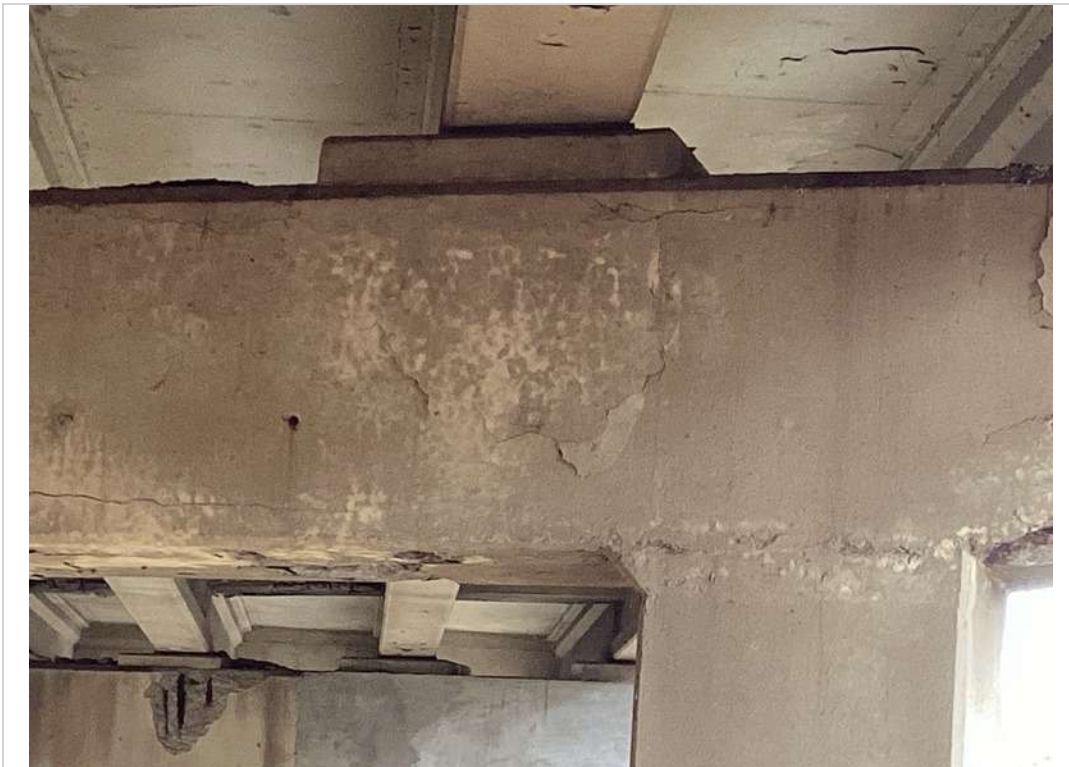
Bent 1 delam on front face of cap under Beam E
