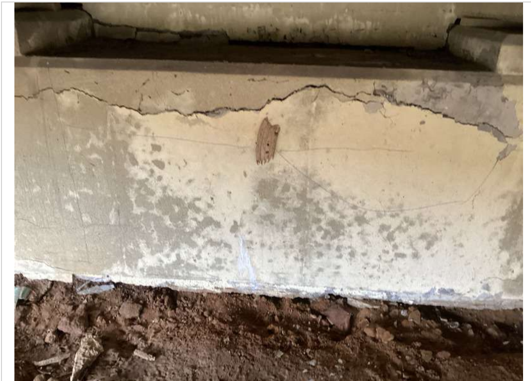
Abutment 1 delam on cap under Bay D
