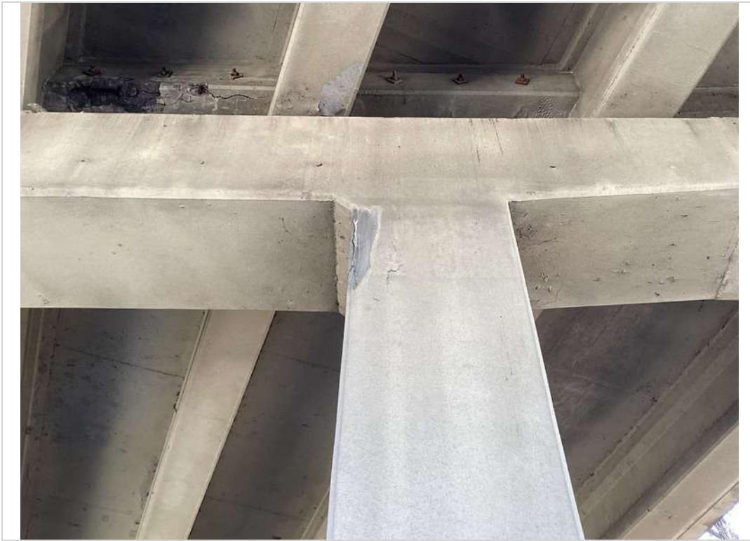
Bent 2 delam in back face of Column B
