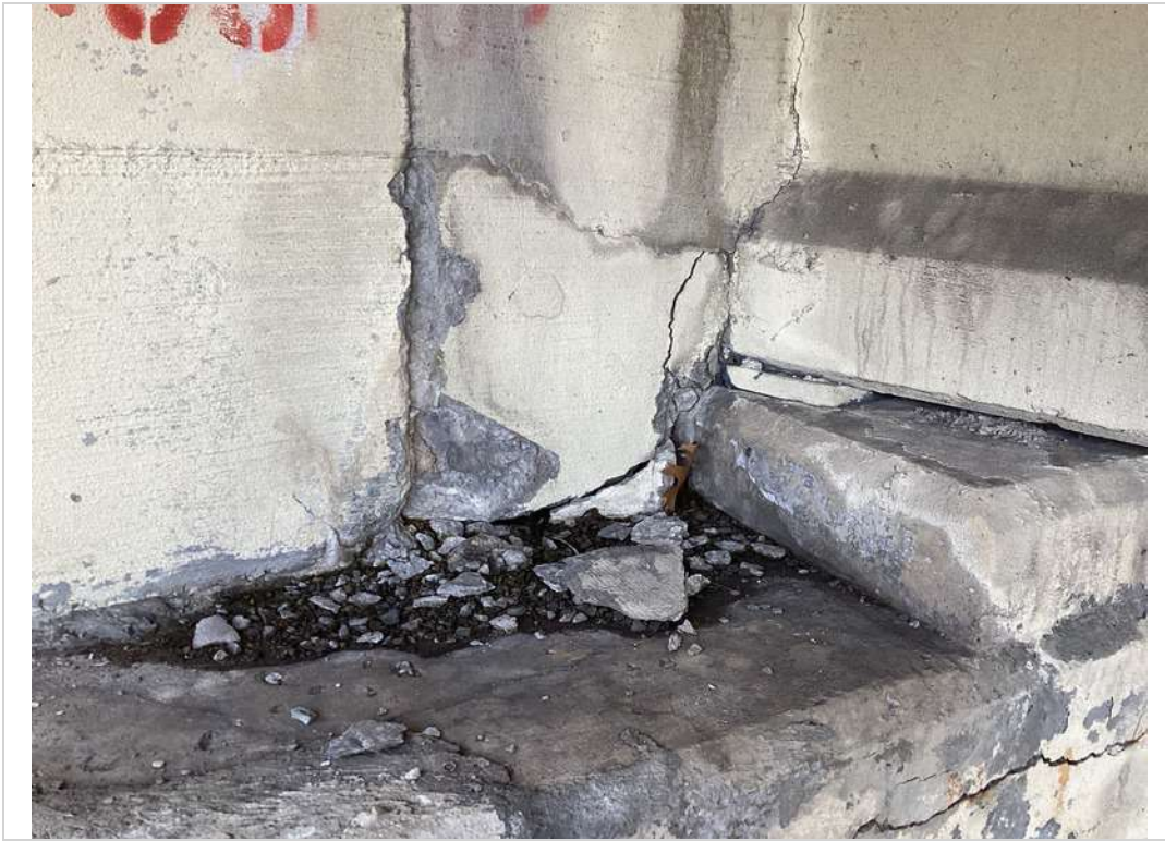
Abutment 1 spalls on backwall under right overhang
