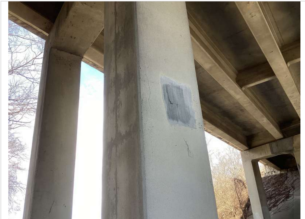
Bent 2 1/32" crack and failed patch on right face of Column B
