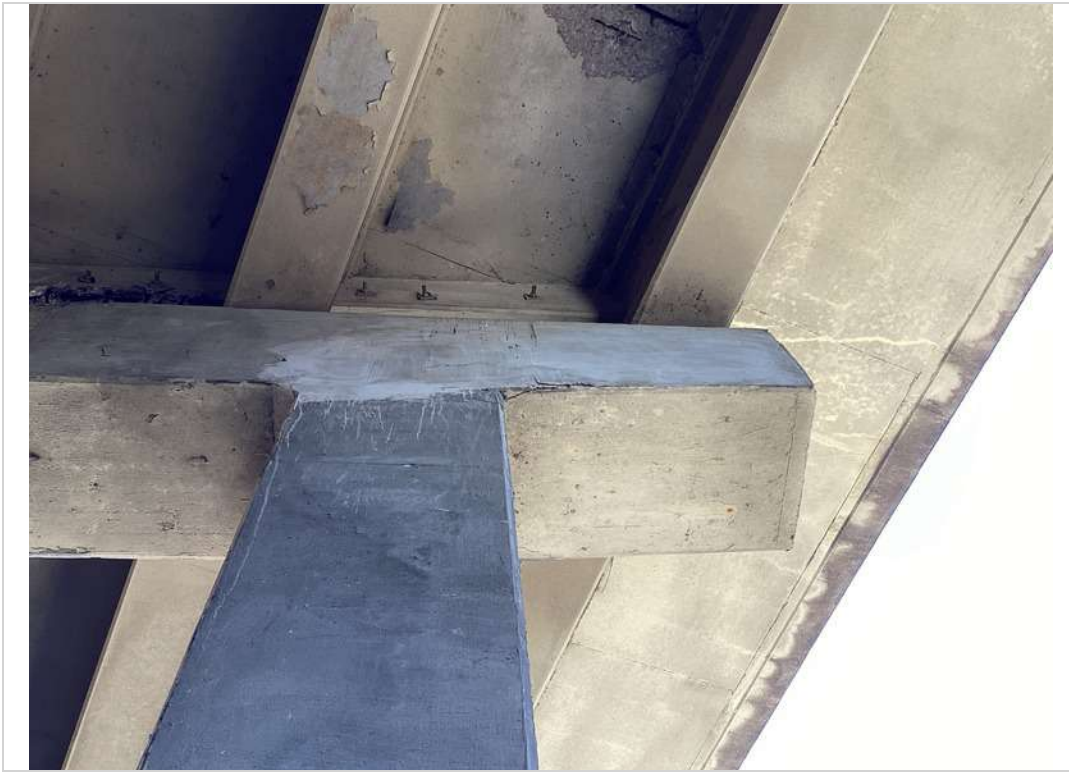
Bent 2 delam in cap above column C
