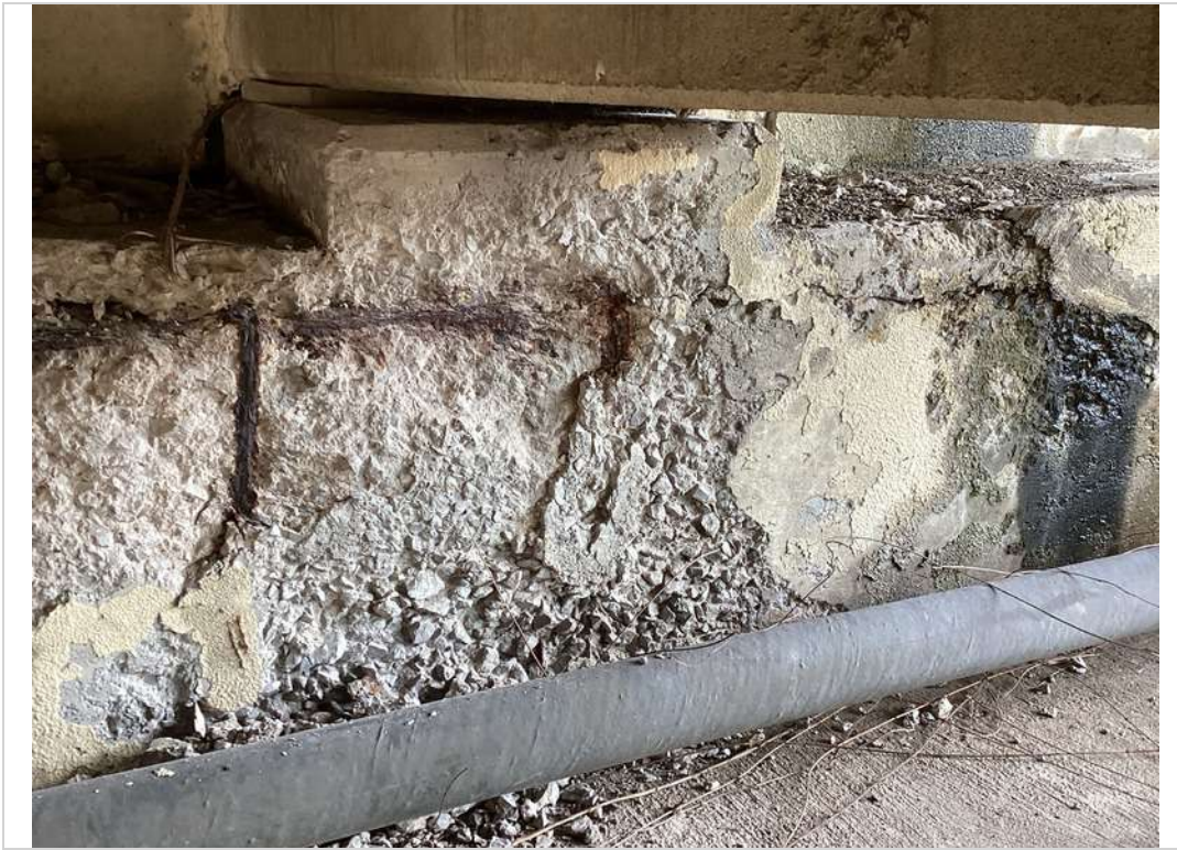
Abutment 2 spalling w/ exposed rebar on cap under Beam E
