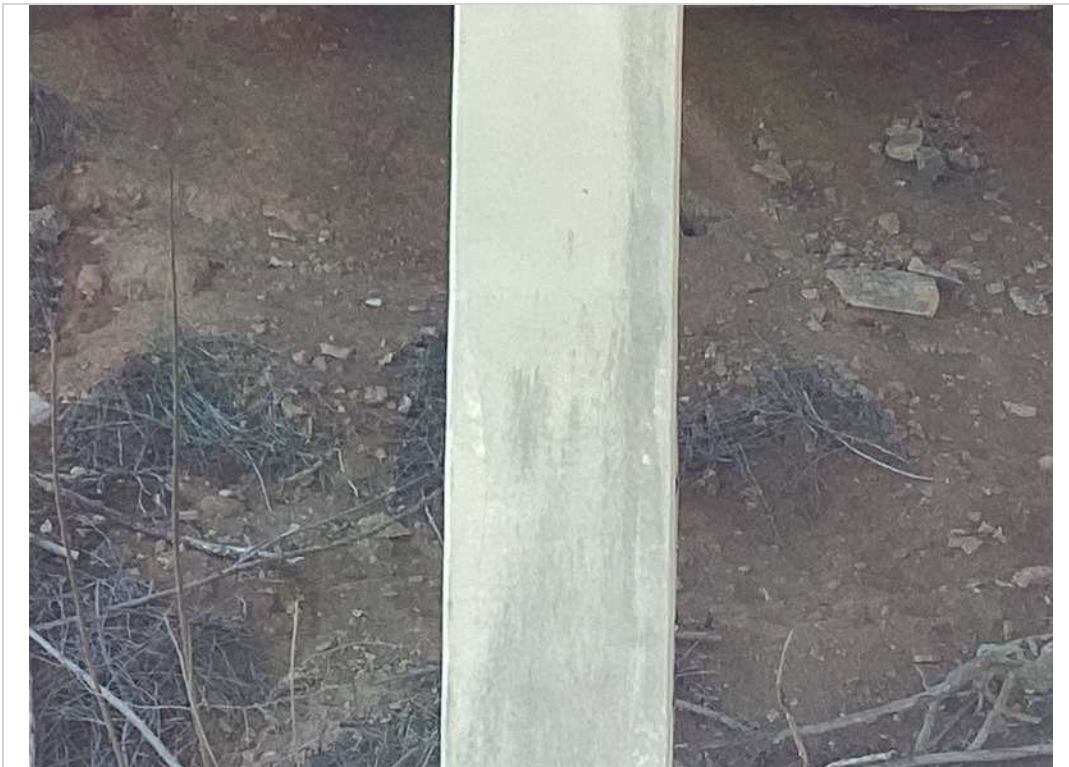
Bent 1 HL crack in Column C
