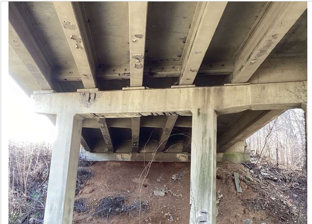
Span 2 spalling w/ exposed rebar and delams in back diaphragms
