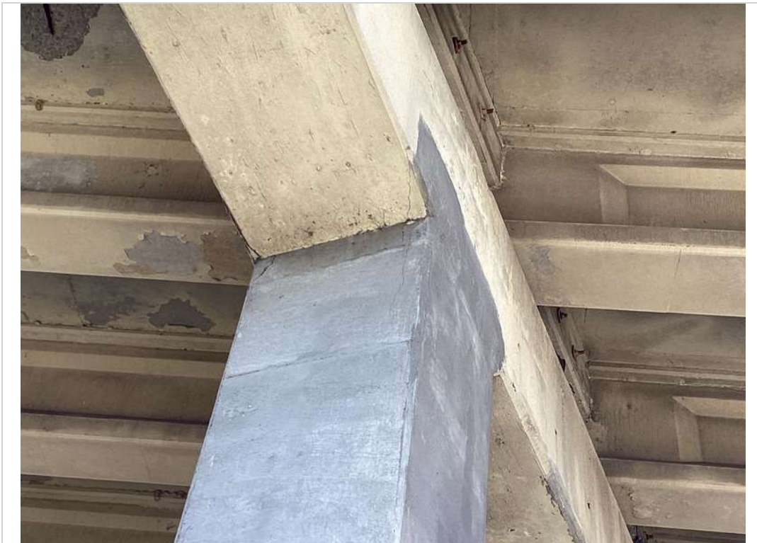
Bent 2 1/32" cracks in right face of Column C
